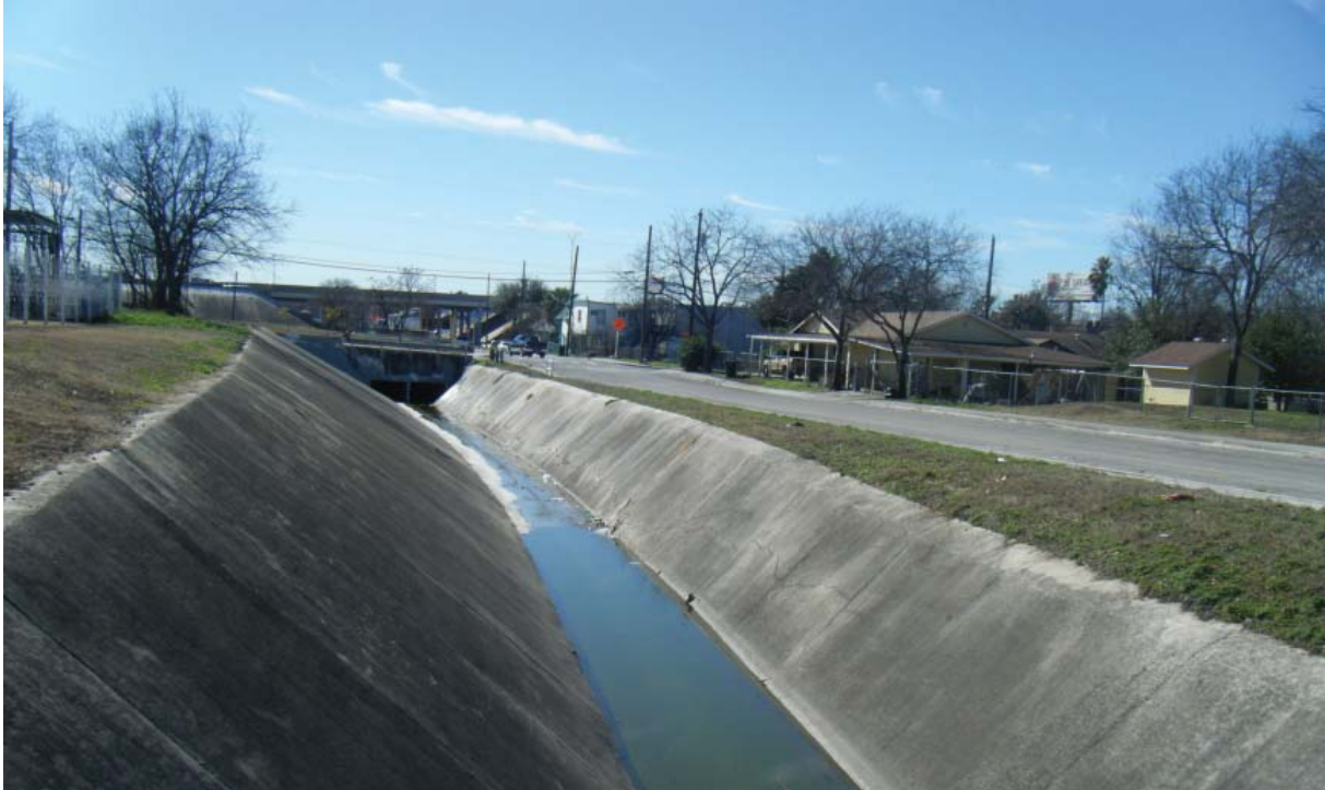
Figure 4. The drain begins at Fort Sam Houston and extends southwest to Sandmeyer Street (view southwest from the intersection of East Carson and Frank Streets).
