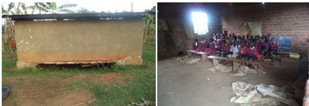
Figure 3: A Collapsing Toilet and an Incomplete Classroom Block at St Kizito-Ggolo Primary School, Ggolo, Nkozi Sub-county
