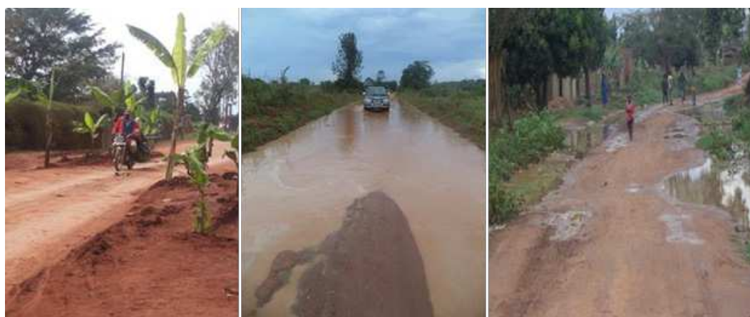
Figure 5: Poorly maintained Roads. Right: Kayabwe – Bukasa Road. Centre and Left: Sections of Kituntu – Kayabwe Road
