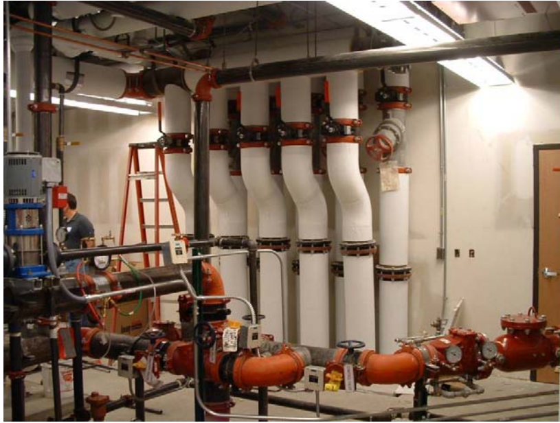
Figure 3. Photograph of the main mechanical room at the Murray High School, showing the ground loop field supply and return headers.
