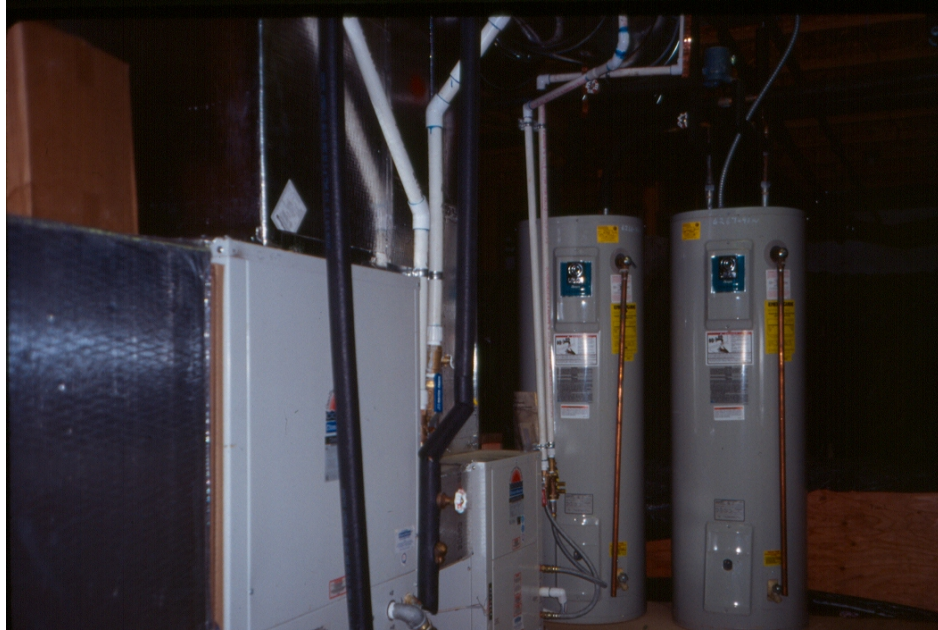
Figure 3. Water to water heat pump.
