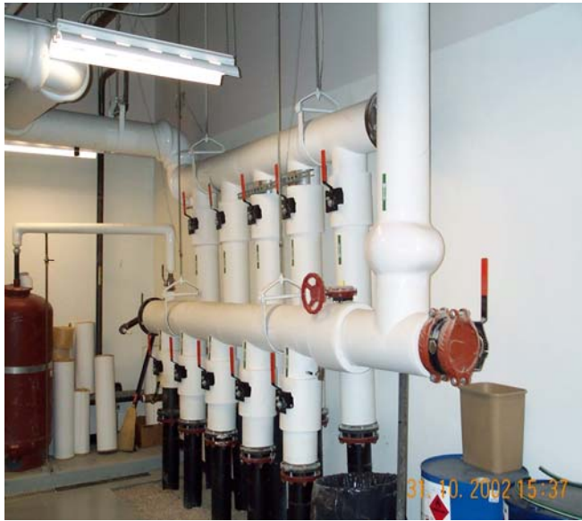
Figure 3. Photograph of the mechanical room at the Canyon View High School, showing the ground loop field supply and return headers.
