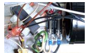
Transformer and fuses.
