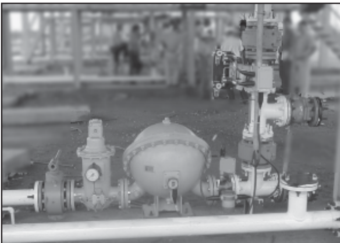
Proper Meter Installation
