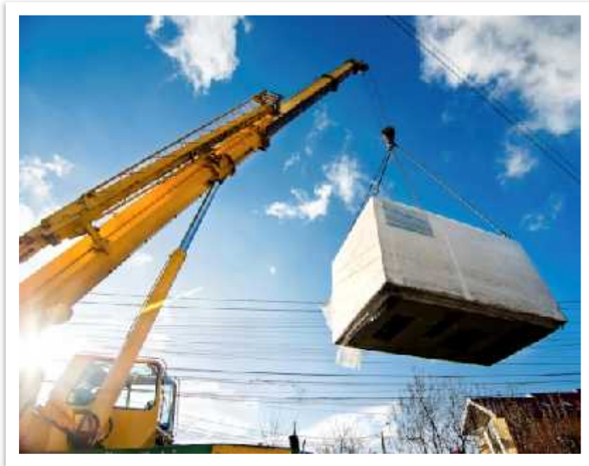
Free fall of the load line hoist is prohibited.
