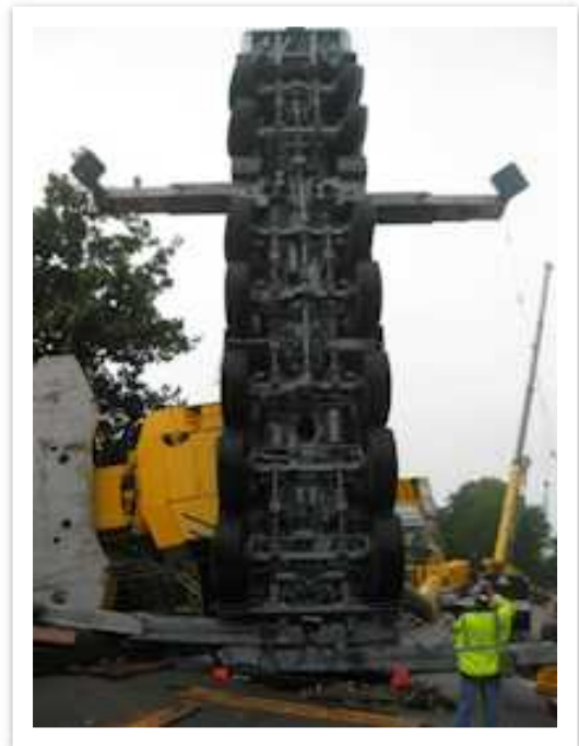
Collapse of equipment caused by exceeding the crane's rated capacity.
