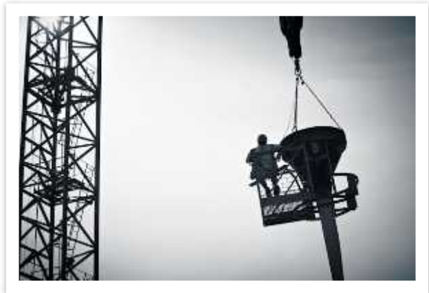
The personnel platform must be equipped with a guardrail system which meets OSHA criteria.
