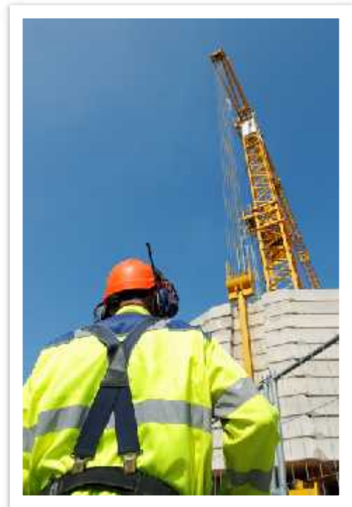
A crane operator often needs a signal person, to be able to operate safely.
