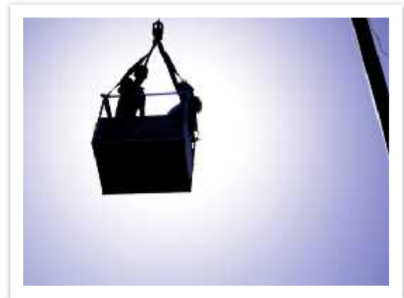
The operator-in-training cannot operate a crane if the crane is used to hoist personnel.
