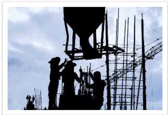
Live booms cannot be used if there are any employees in the fall zone of the boom or load.
