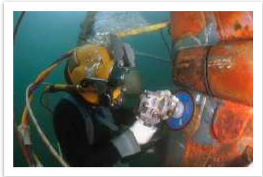
When a crane is lifting a diver, it must not be used for any other purpose until all the divers are back on board.
