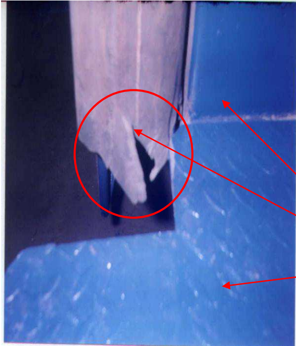
Figure - 1.5 Rubber flange torn by foot plate. and buffer to Drg. no. RDSO SKETCH -88050.
