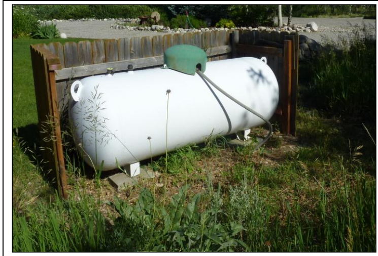
Lack of proper clearance can compromise the integrity of propane storage tanks and place both the homeowner and first responders at risk.
