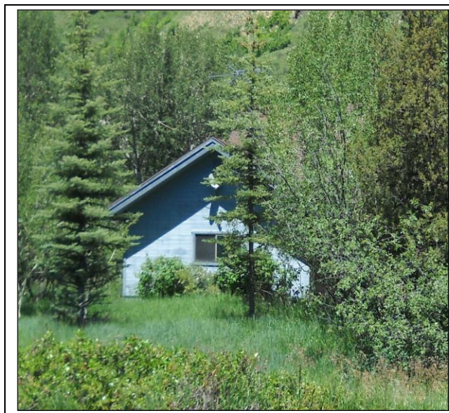
Lack of mowing and ornamental shrubs against the house will almost assure the ignition of this home in a wildfire.
