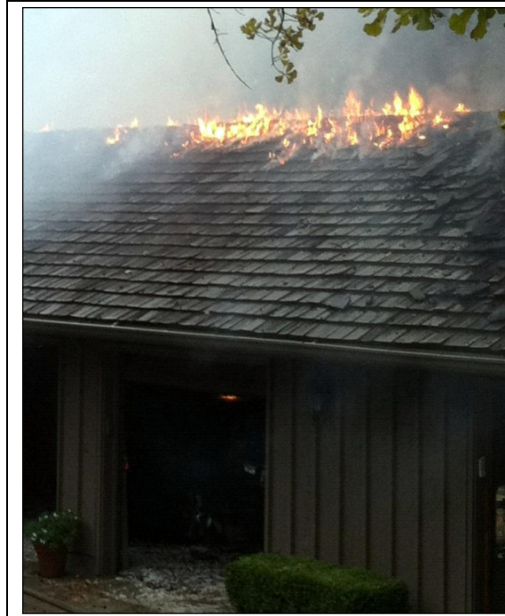
In a wildfire situation a wood shake roof is almost guaranteed to ignite.
