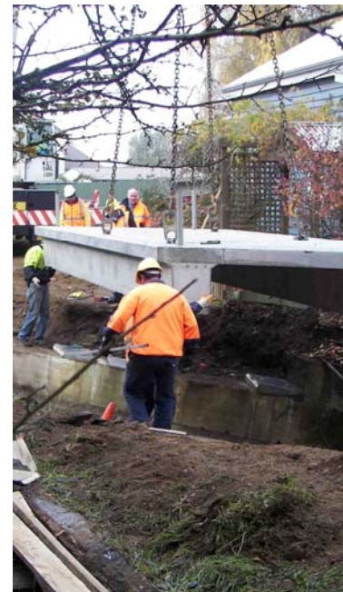
The Council's bridge crew replaces a bridge as part of the Council's 2009/10 Bridge Replacement Program.
