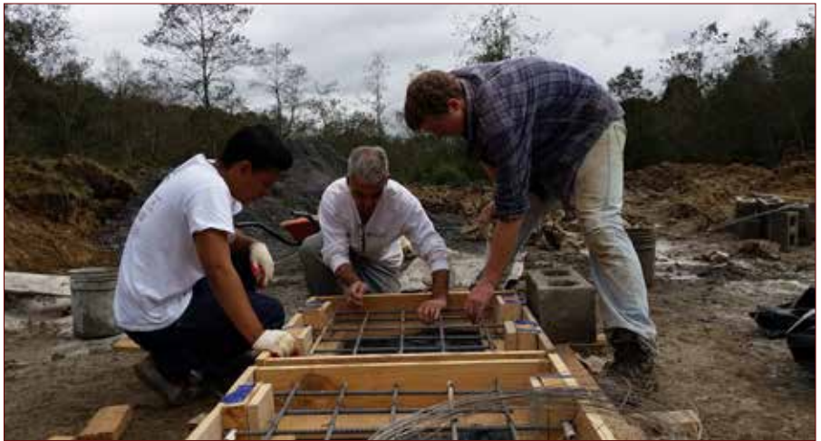
Civil engineering student Marvin Merida, civil engineering alumnus and Engineers Without Borders mentor Rick DiSalvo, and mechanical engineering student Joe Buellesbach work on hatches for a septic tank in Xix, Guatemala.
