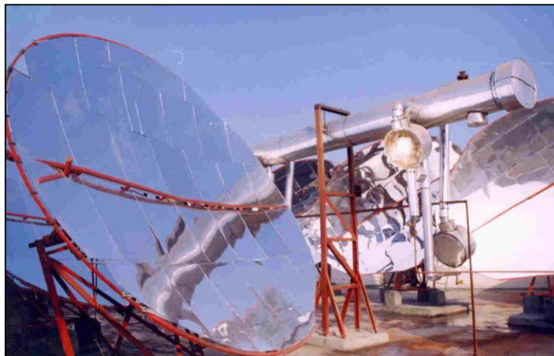
Figure 3.1: A Scheffler solar dish for steam generation
