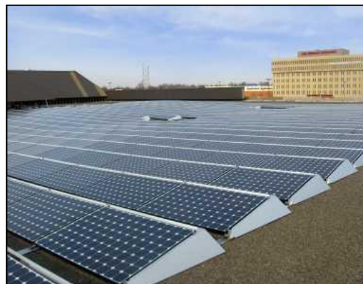
Building Integrated Solar PV on Roof
