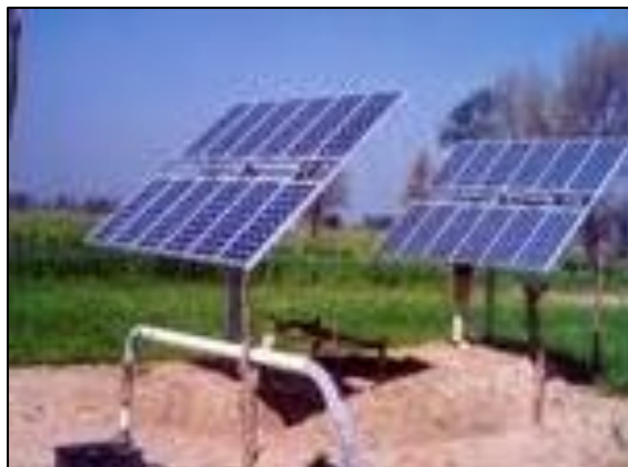
Figure 2.1: Stand-alone PV for water pumping in field
