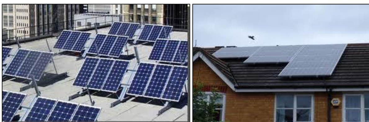
Figure 2.6: Roof top PV
