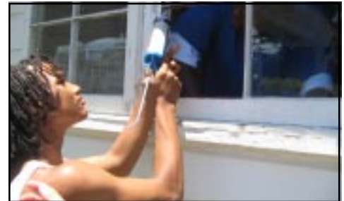
Akeem McDay, Asheville Water and Energy for Justice Youth Team, caulks a leaky window
