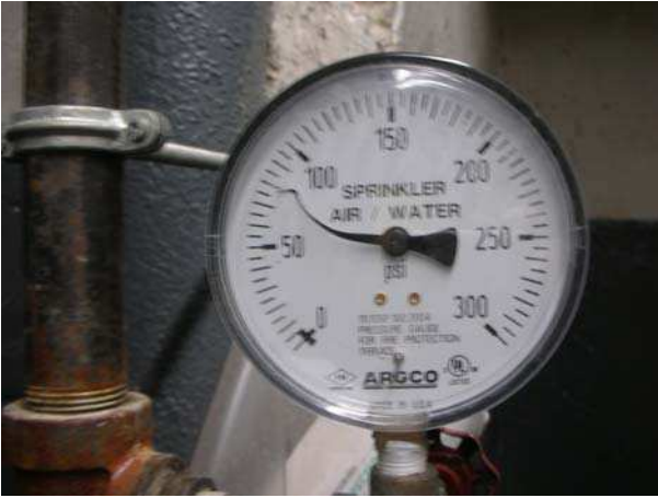
Defective Water Pressure Gauge
