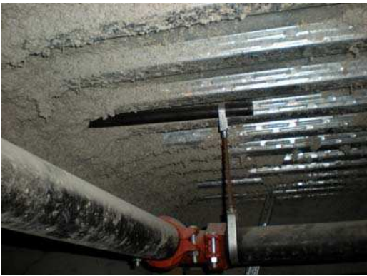
Sprinkler System Improper Hanger
