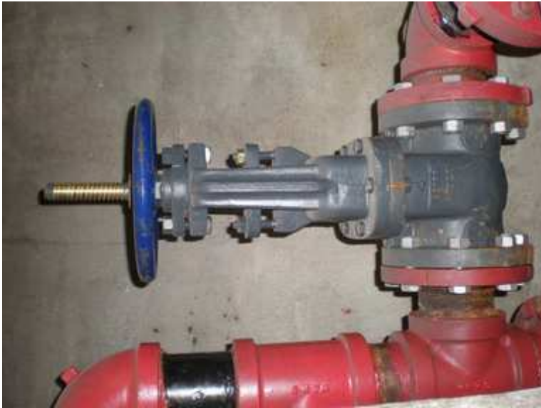
OS & Y valve Not Sealed, Locked, Electronically Monitored, Labeled and Valve Handle Not Painted
