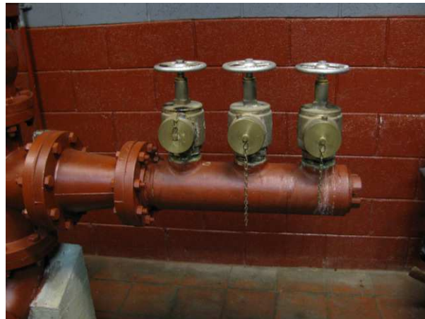
Fire Department Test Manifold
