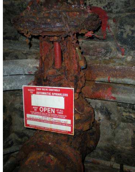
Corroded Curb Valve in Sidewalk Vault
