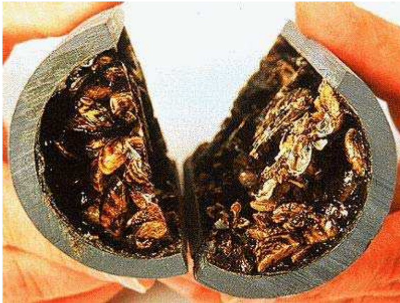
Piping Infested with Zebra Mussels
