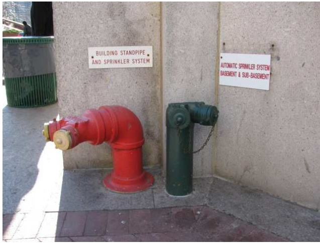
Sprinkler & Standpipe Fire Department Connections
