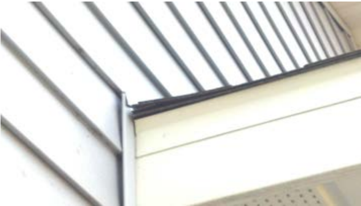
"Kick out" flashing should be at the bottom of all exterior roof to wall intersections to help divert water from entering behind siding.
