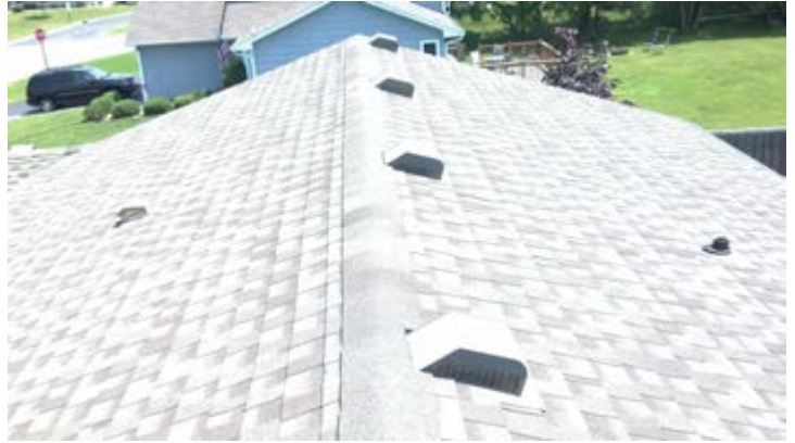
Recommend additional ventilation. Plumbing stacks do not extend far enough above roofline- recommend repair as necessary. Plumbing stack boots are not properly sealing around plumbing stacks making them vulnerable to exterior conditions- Recommend repair as necessary.
