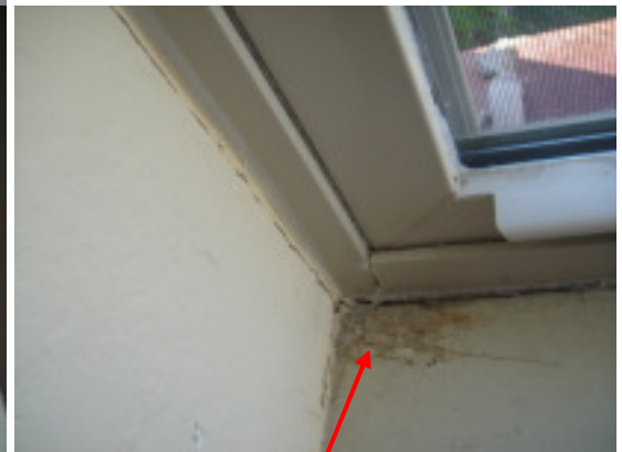
Water stain on window sill in upstairs south bedroom.
