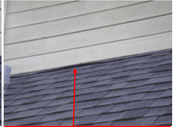
Shingles not secured down properly on the north side of the home.
