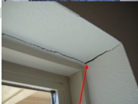
Movement cracks in the master bedroom south window.
