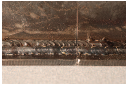
Fig. 5 — Sample of visually acceptable multipass fillet weld with poor fitup and a slugged and bridged root opening that has been welded over as an example. (See Fig. 6.)
