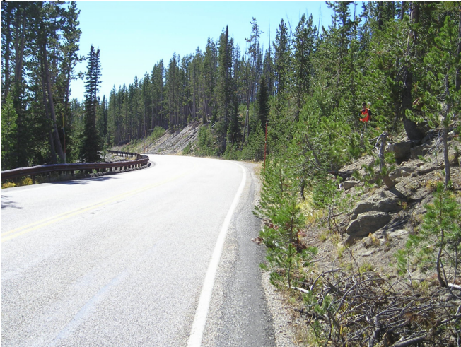
Looking south along highway at bench mark (beneath person) and north end of guardrail.
