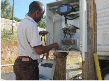
Remote meter reading installed in Petit Goave
