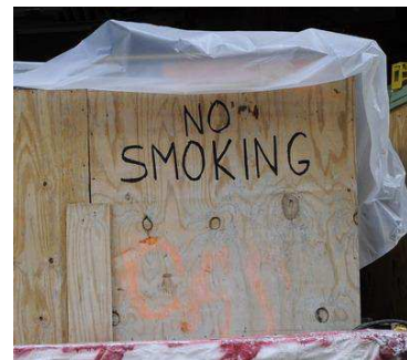
Unacceptable Warning Sign
