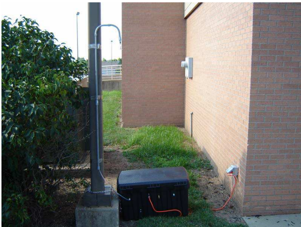
Figure 7. Site 3 Equipment and Setup
