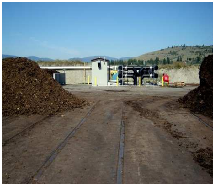
ASP Aeration Equipment
