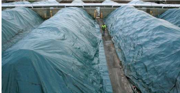
Photo of a GORE covered ASP system
