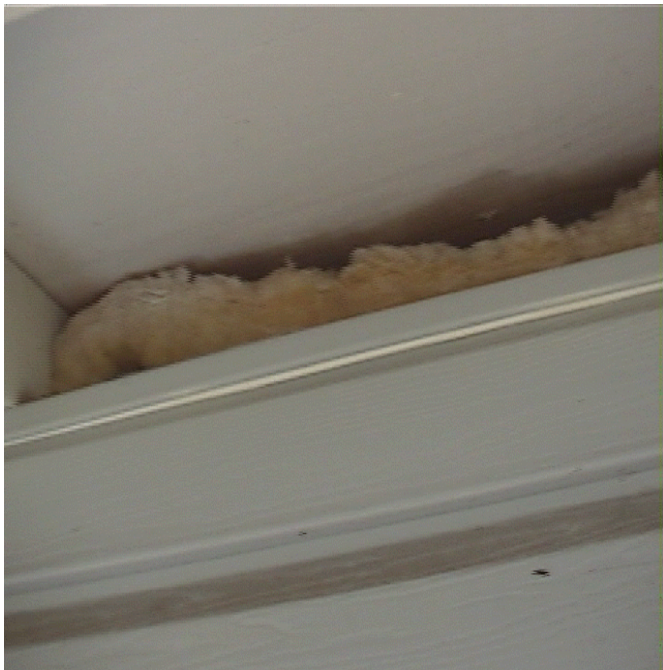
Gap between wall and ceiling creates health hazard.
