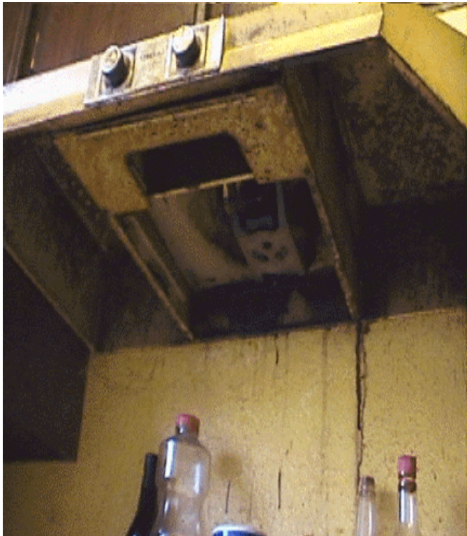
Greasy range hood is a fire hazard. The exposed fan and wiring are electrical hazards.
