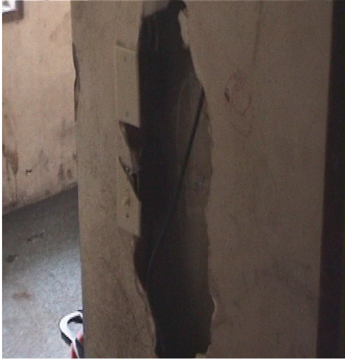
Hole in wall creates safety and electrical hazards.
