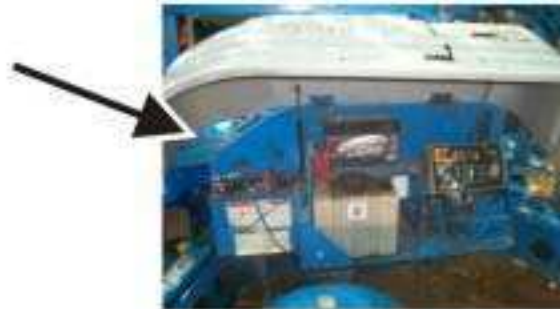
Motor Controller compartment
