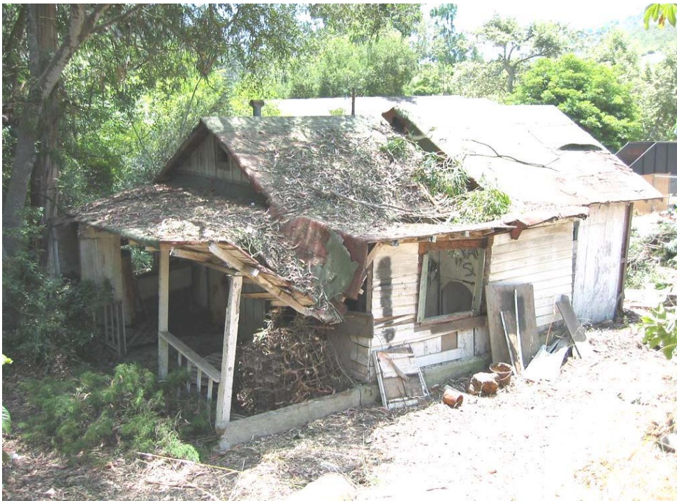
Plate 5. North and east elevations of cabin before porches were removed for repair. Facing south west. 2002. Courtesy Linda Dye
