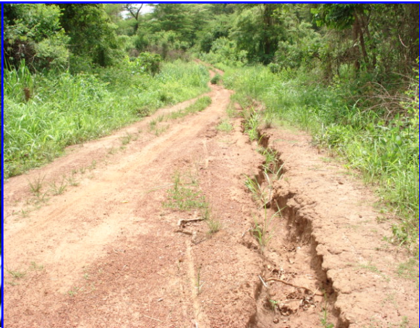
Rutting Formed due to Lack of Drainage
