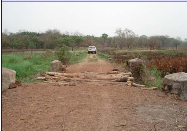
Deck of the Damaged Bridge Replaced with Wooden Logs to Keep Traffic Flow
