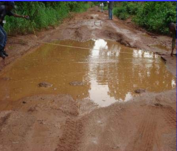
Potholes Formed on the Road
