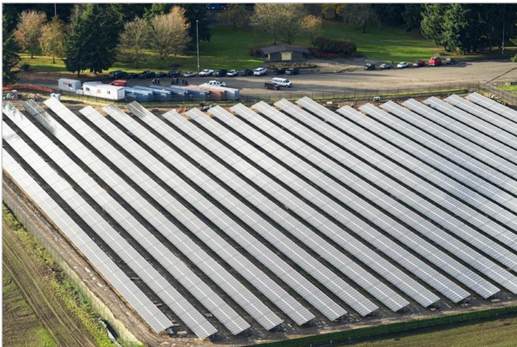
Figure 5: Aerial view of Oregon DOT's Baldock Safety Rest Area Solar Highway Project Photo credit: Gary Weber, Oregon DOT
