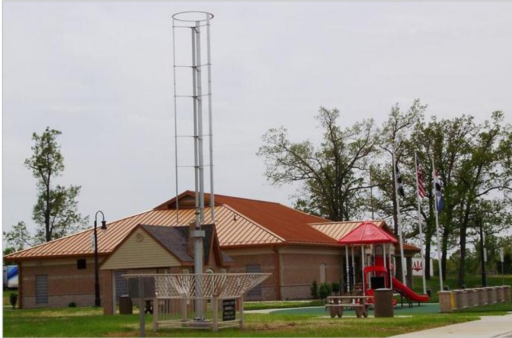
Figure 11: One of two, 1.2 kW wind turbines (one in each traveling direction) installed at Missouri DOT's Conway Missouri Welcome Center on I-44 . The wind turbines power the lights over the information counters.
