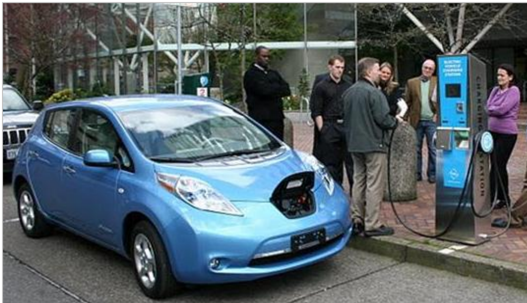
Figure 18: Electric vehicle charging station in Portland, OR Photo credit: Oregon DOT
