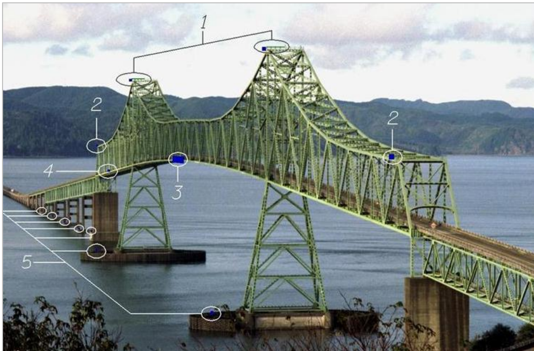
Figure 6: Locations of the five different types of solar lights on the Astoria-Megler Bridge Photo credit: ODOT
