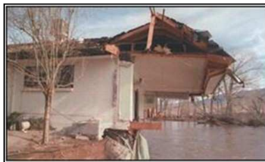
Dangers of channel migration are severe. This home in the Dayton Valley was torn apart when banks were eroded by the force of floodwaters in the incised channel. (Marihyn Newton, Reno Gazette Journal)
