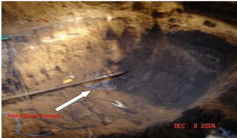
Figure 1 - Gas burning in bell hole
