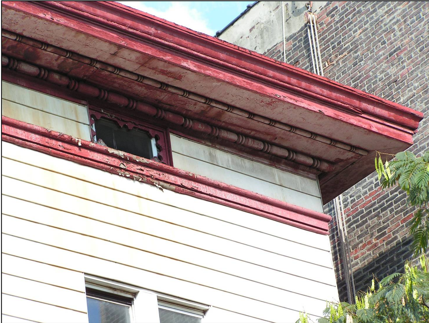
George B. and Susan Elkins House, cornice and attic window details. Photo: Michael Caratzas
