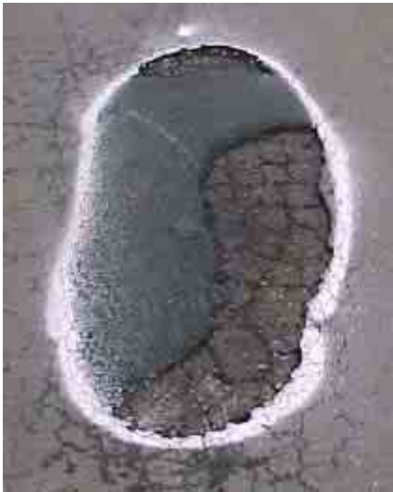
Figure 4.9: Albany mix partial failure
