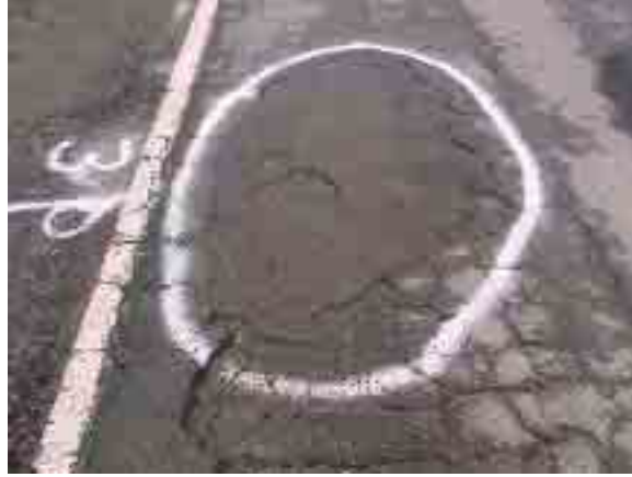
Figure 4.11: Instant Road Repair failure after one week
