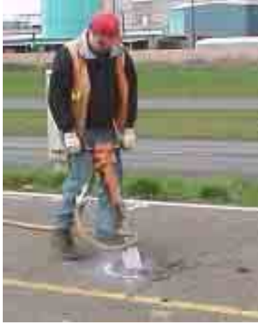
Figure 4.1: Manufacturing a pothole at Century Drive
