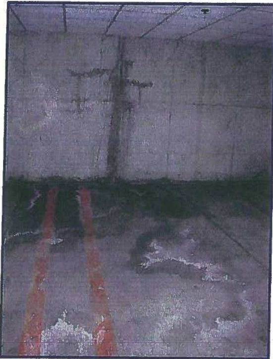
Photo 11. Active foundation wall leak @ Basement level
