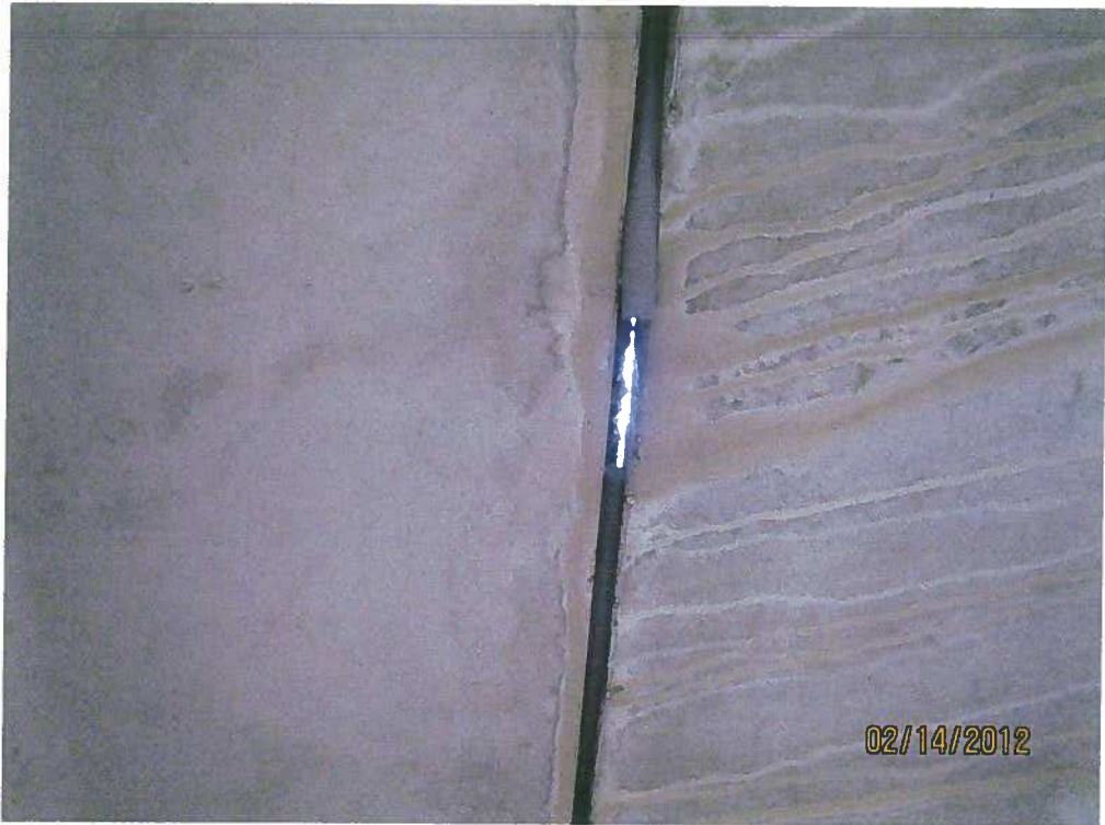
Underside of 6th Level Parking Garage Sealant Joint EXHIBIT 'C'
