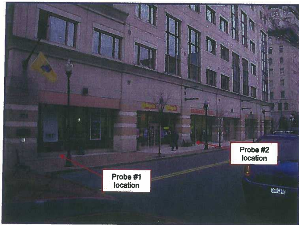
Photo 2. North elevation of building west of the main entrance along East State St.
