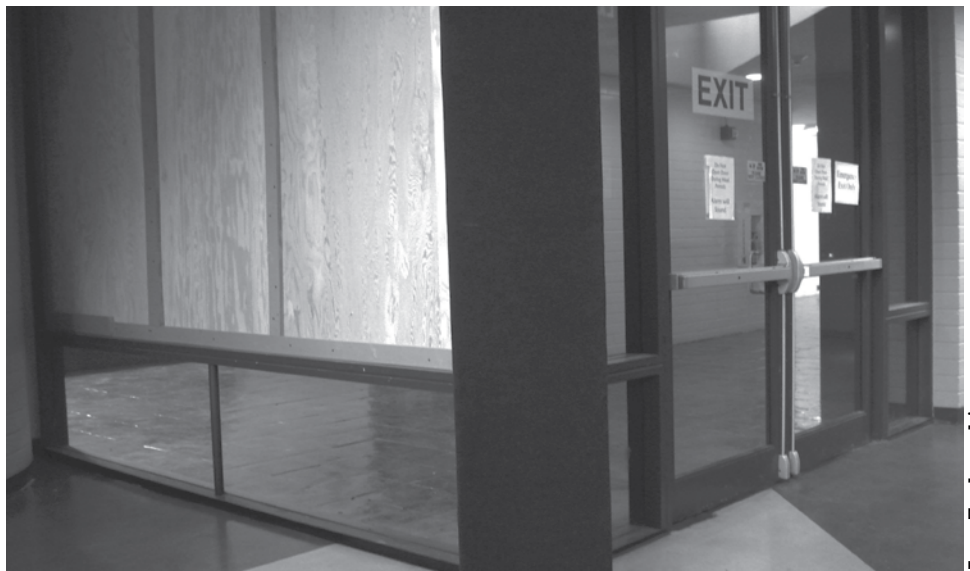
The boarded up window in the Dining Hall.
