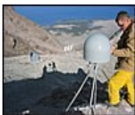
GPS receiver installation
