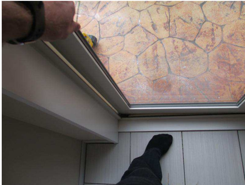
Figure 5 – some evidence of movement in external lounge door
