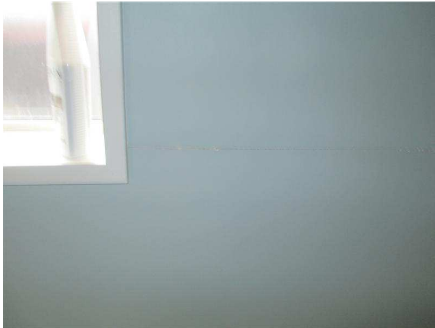
Figure 7 - Horizontal crack in Gib lining in ensuite
