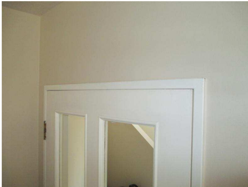
Figure 8 - Slight twist in internal door frame - door still opens and shuts
