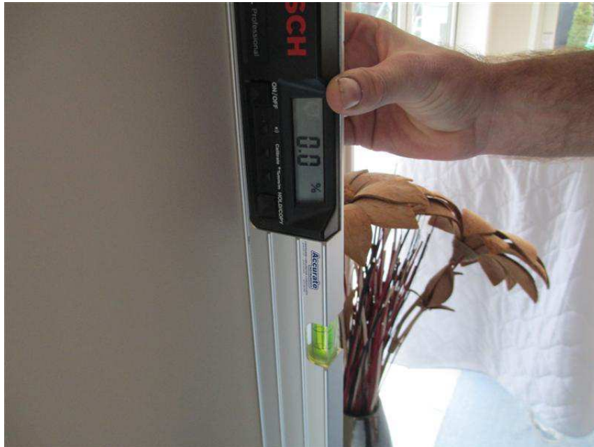
Figure 9 - Level checks on both ground and upper floor were generally good, minor lean to the northeast
