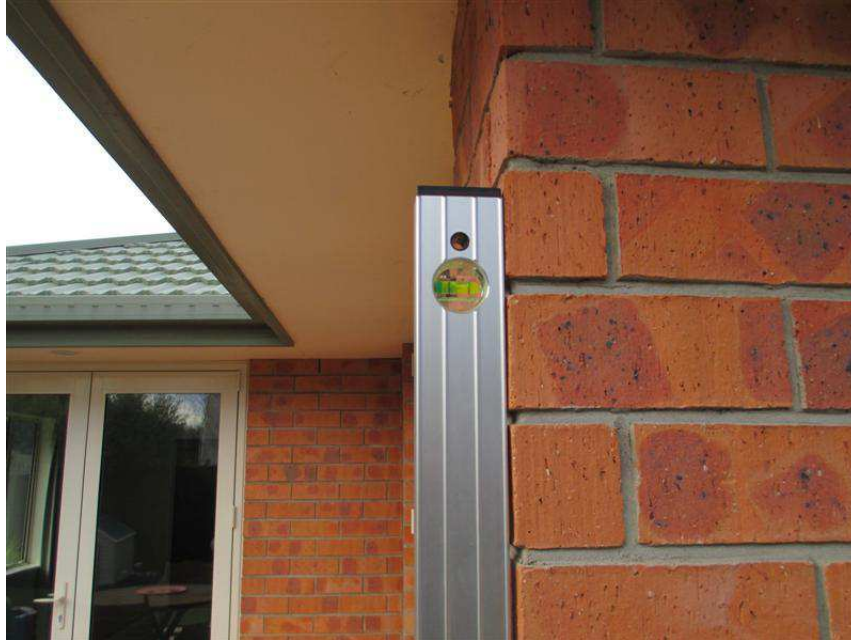
Figure 3 - External wall checks revealed minor lean to the northeast
