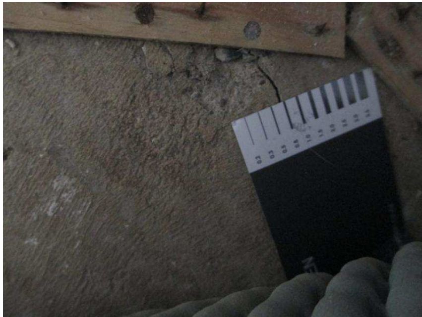
Figure 6 - Crack in lounge floor slab (up to 0.6mm)
