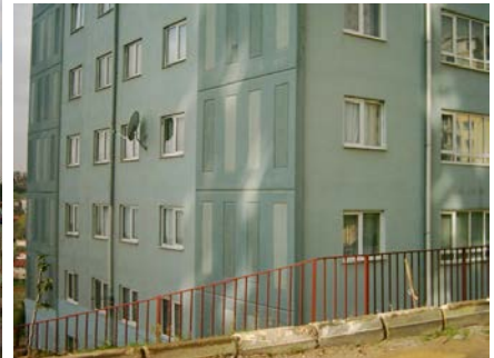
Figure 18: This Tunnel Form Building Located in Bekirpasa/Izmit Also Suffered No Damage during the Earthquakes in 1999
