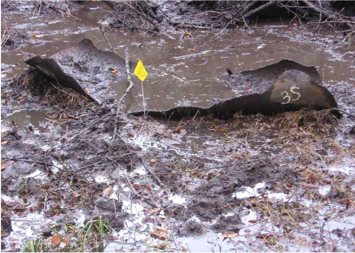
Figure 3: Severed 9 foot section of pipeline
