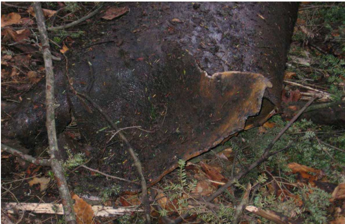
Figure 2: Severed 37.1 foot section of pipeline
