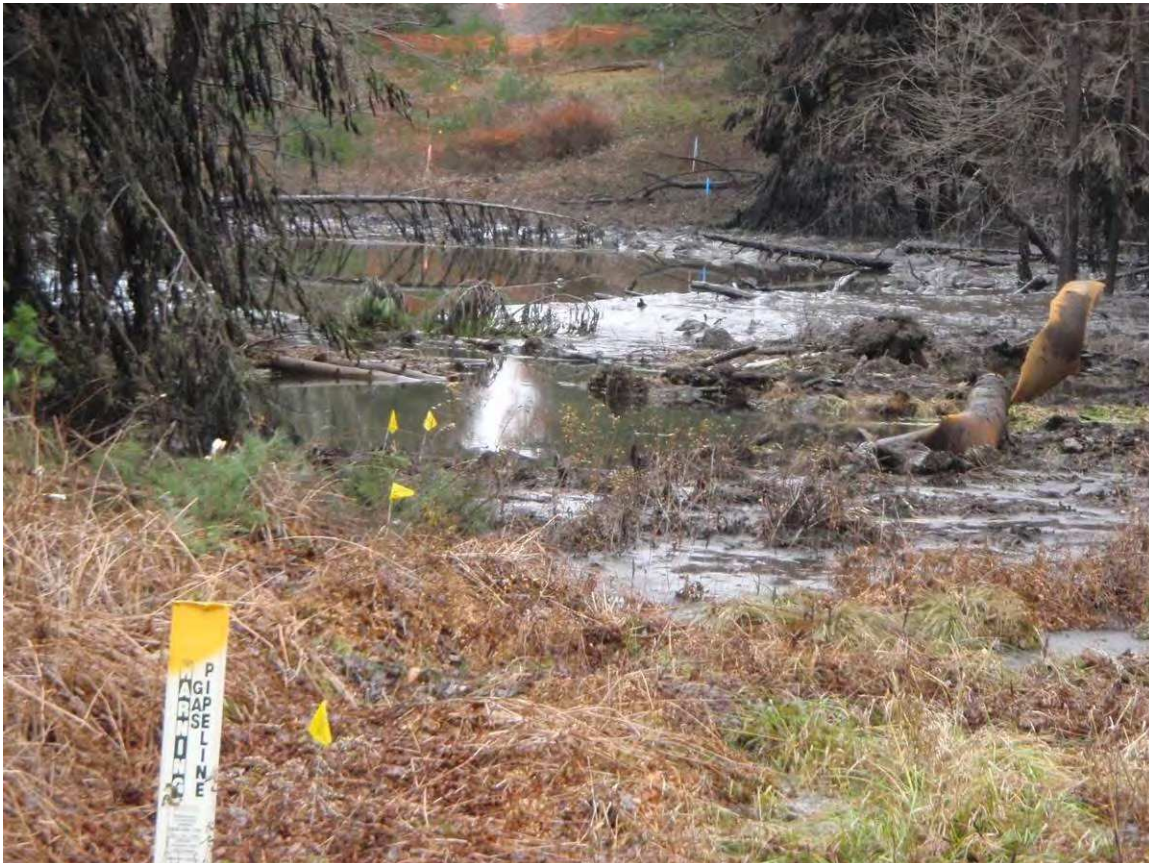
Figure 8: Ruptured pipe in swamp
