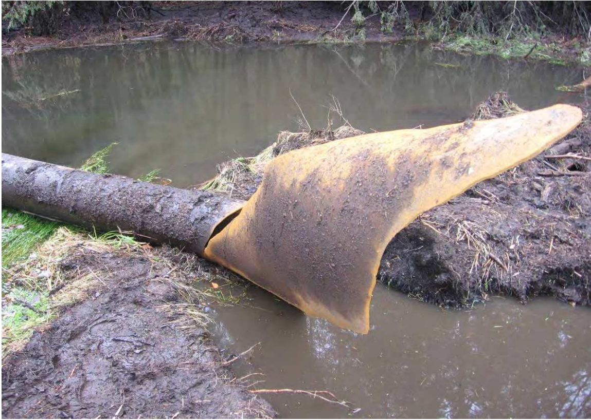
Figure 5: End of severed 37.1 foot section of pipeline
