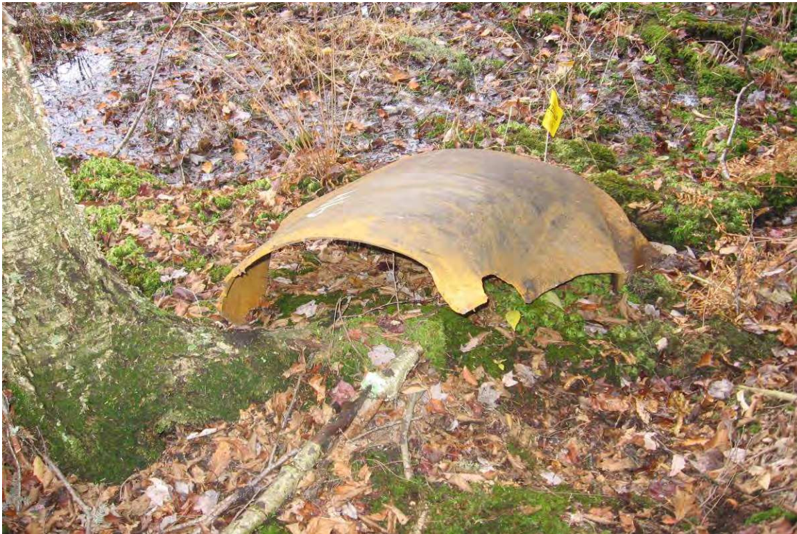
Figure 4: Severed 4.7 foot section of pipeline, piece 4
