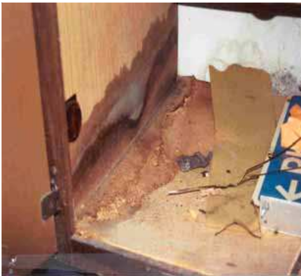
Sink cabinet sides and bottom shelf rotted out at Saraland Manor Apartments.
