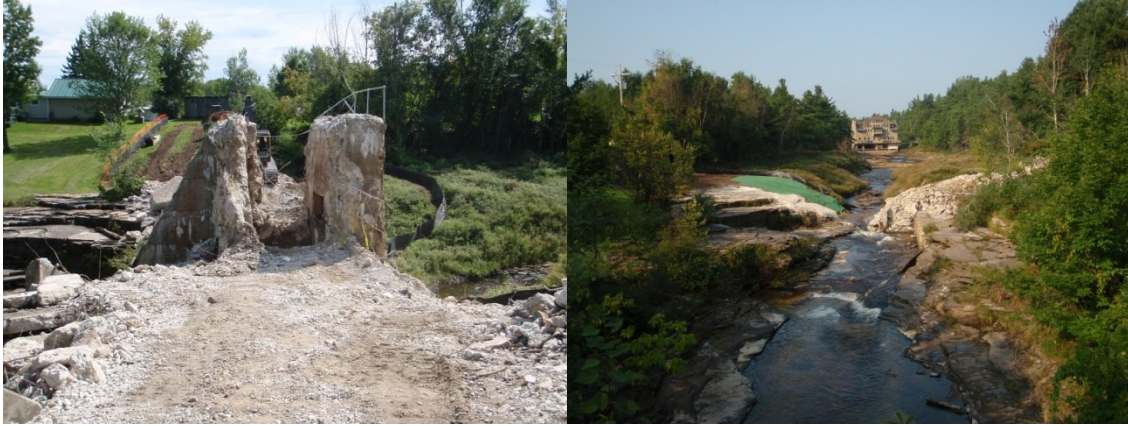
LaSalle Dam on the Great Chazy River in Town of Altona, (Clinton County, NY). The left picture was taken of the dam before its removal on August 23, 2010. The right picture shows stream corridor on September 1, 2010. The failing dam was a barrier to fish and navigation. Its removal eliminated a public safety hazard and reduced local flooding. Photo credit: DEC Region 5
