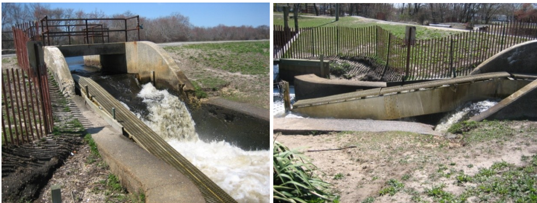
Views of the seasonal Alaskan Steep Pass Ladder along the left approach up the North Spillway in Grangebel Park. This is along the Peconic River in the Town of Riverhead NY in Suffolk County. The ladder, installed every spring since 2000, re-opens 1.5 miles and 24 acres of diadromous fish habitat. A permanent rock ramp was installed in the other spillway in 2010. Photo credit: DEC Peconic Estuary Program
