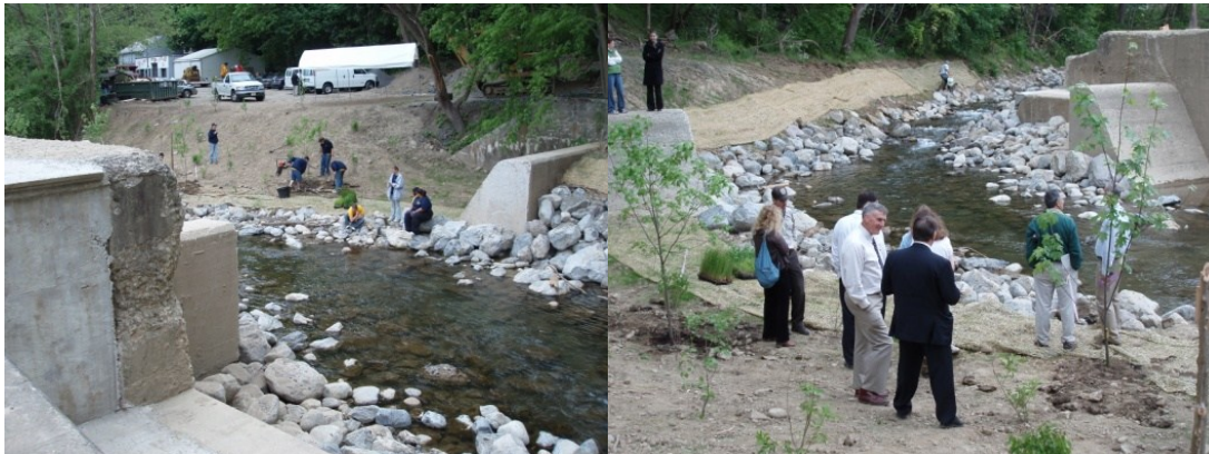
Partial dam removal at the Pursel Mill Dam on Lopatcong Creek in Phillipsburg, NJ. Portions of the spillway and abutments were retained for historic purposes. Photo credit: American Rivers
