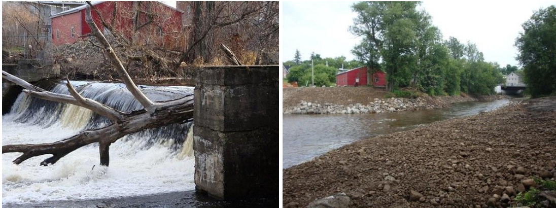
Fort Covington Dam on the Salmon River in Fort Covington (Franklin County, NY). The dam was removed June and July 2009. The deteriorated 10-foot dam was a barrier to fish and navigation. Its removal eliminated a public safety hazard, reduced local flooding and opened up more than 35 miles of river for migratory and resident fishes. Photo credit: Town of Fort Covington
