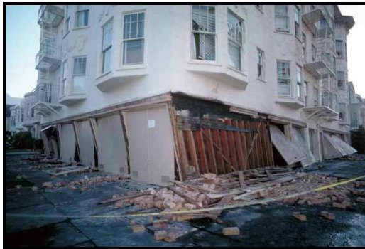
Damage to Housing in 1989 Loma Prieta Earthquake
