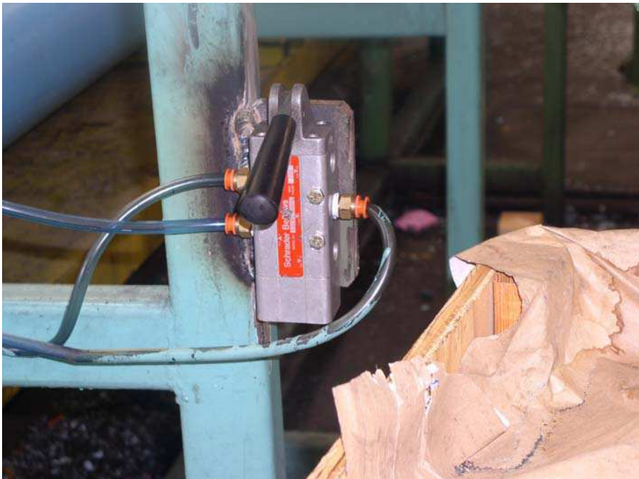
Exhibit 4. The switch used to activate the pipe storage rack stoppers.
