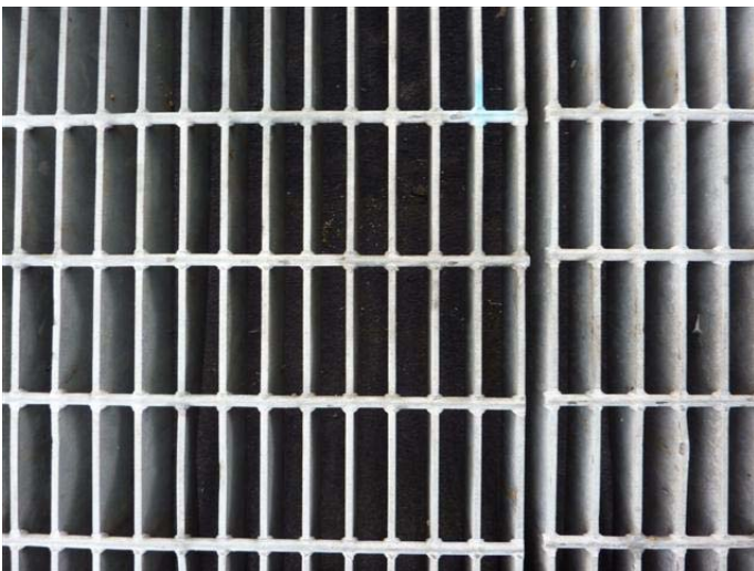
Photo 3. Screened storm drain, obstructed with debris. Plastic dust and particles are visible on the ground and in the drain.
