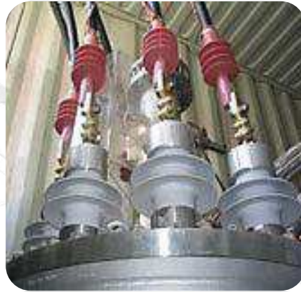
Superconducting Fault Current Limiters (SFCL)
