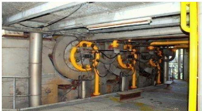
Figure 2.7: Burner used in 150 MW & 15.75 KV of APSCL.
