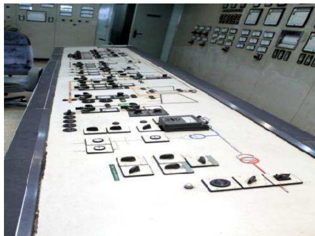
Figure 2.21: Analog control system in a control room of 64 MW & 11 KV unit 1.
