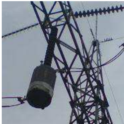
Figure 5.21: Wave trap used on APSCL substation.
