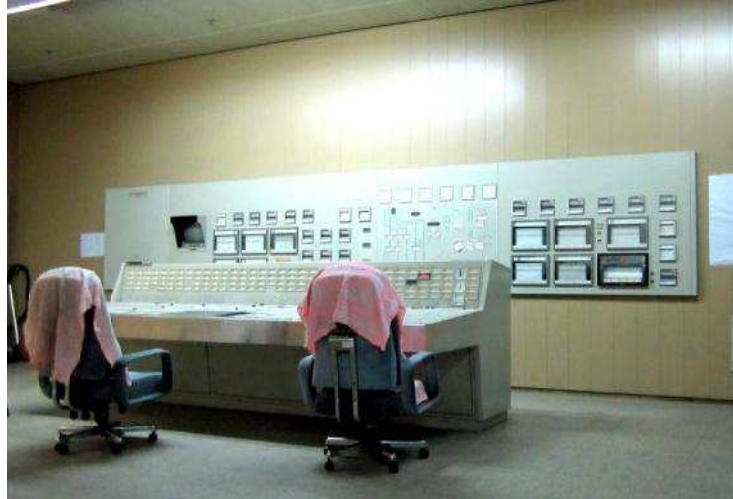
Figure 2.22: PLC controlled control room in 150 MW & 15.75 KV unit 4.
