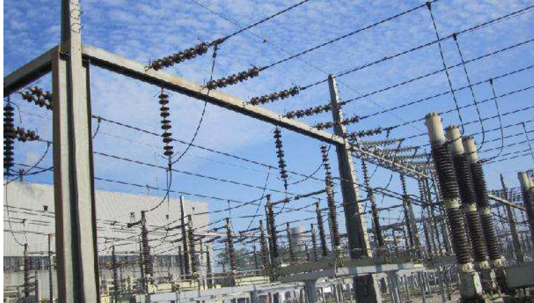
Figure 5.28: 230KV Double circuit bus bar.
