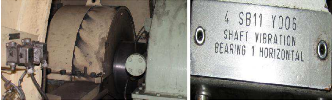
Figure 4.8: Shaft vibration sensor for unit 5 steam turbine connects with shaft.
