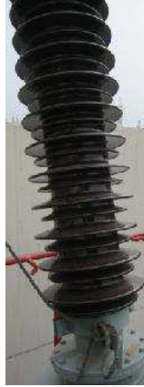
Figure 5.5: Bushing of power transformer.
