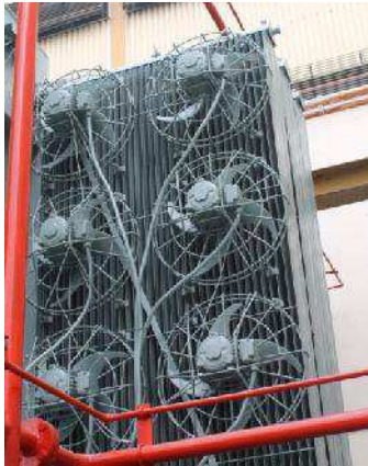
Figure 5.3: Radiator of a power transformer.
