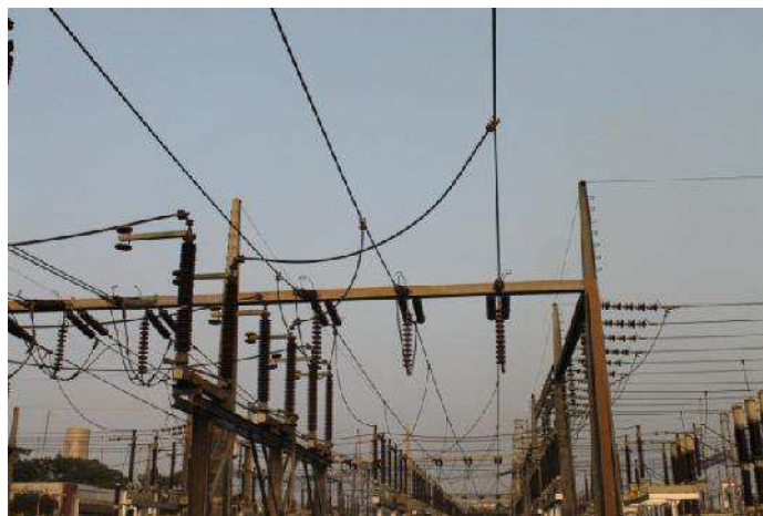
Figure 5.16: 132KV double circuit bus bar.
