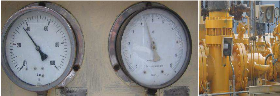
Figure 3.1: Gas pressure reducing valve.
