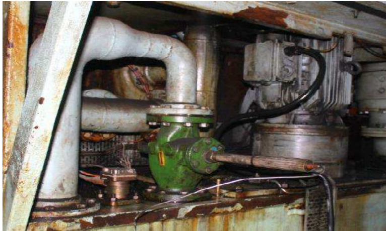
Figure 2.3: Jacking oil pump in 36.7 MW generator of CCPP.
