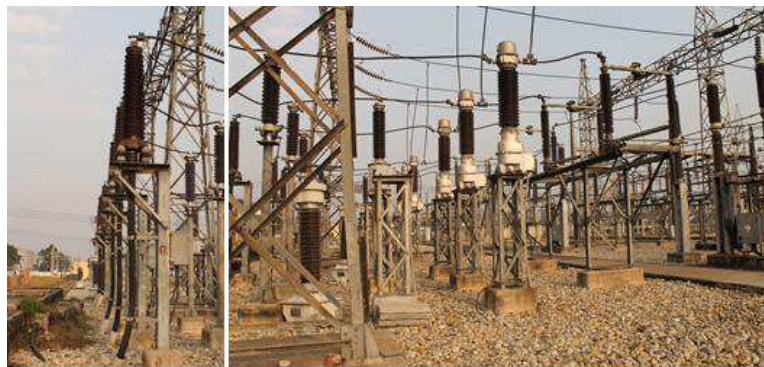
Figure 5.27: Typical 230KV feeder for unit three.
