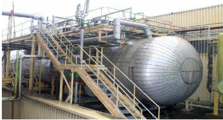
Figure 2.16: Deaerator in 150 MW & 15.75 KV unit 3 at APSCL.
