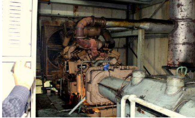
Figure 2.17: Diesel engine in 56 MW & 13.8 KV GT of CCPP.
