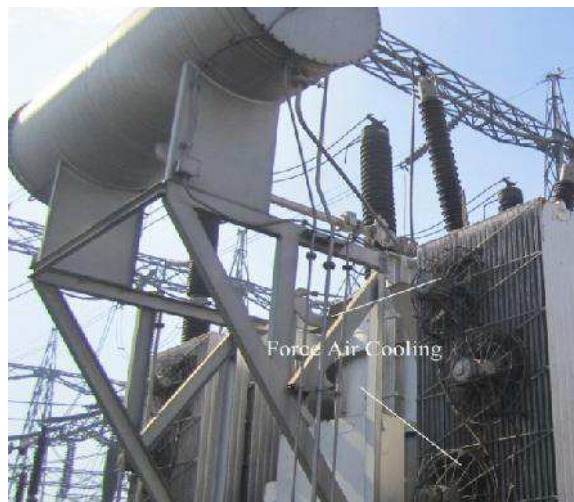
Figure 4.17: Forced air cooling system of transformer.
