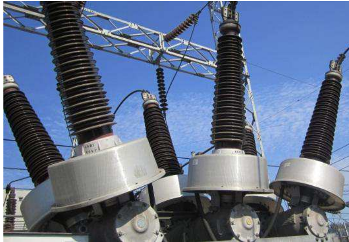
Figure 5.12: SF6 circuit breaker.
