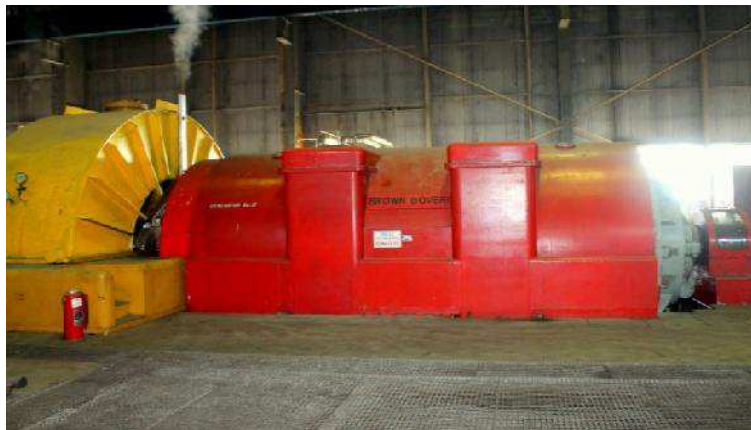
Figure 2.1: 150 MW AC generator of unit 3 .
