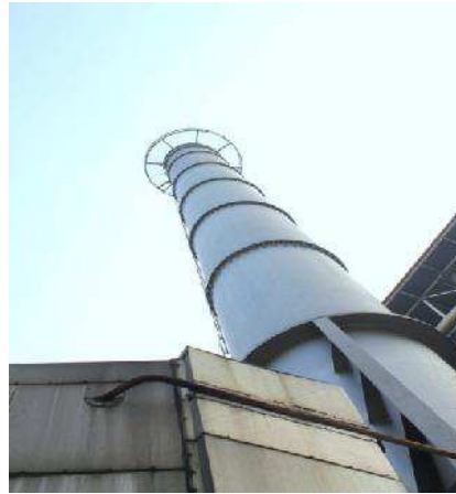
Figure 2.14: Chimney in 64 MW & 11 KV units 1.
