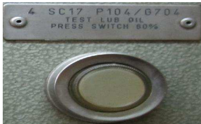
Figure 4.9: Lube oil pressure control switch.
