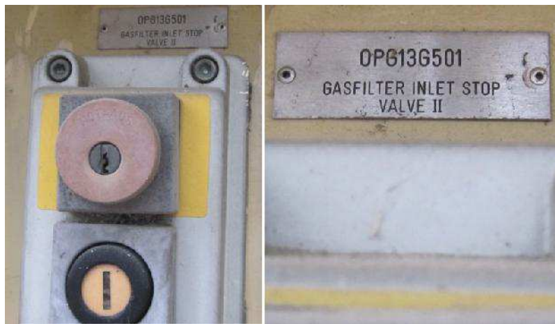
Figure 3.2: Gas filter inlet shut off valve.
