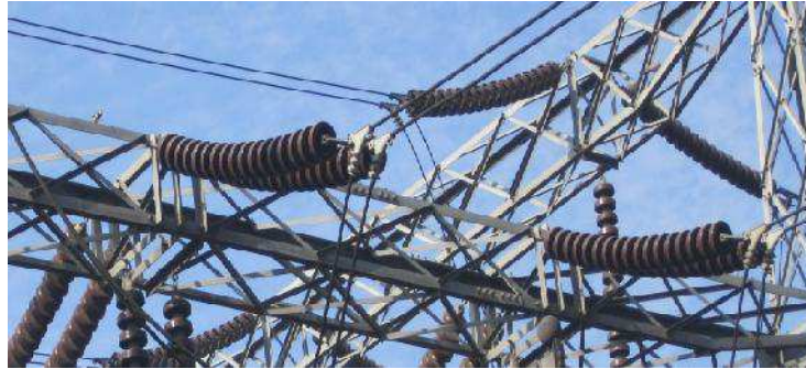
Figure 5.18: Suspension type insulator observed from APSCL substation.
