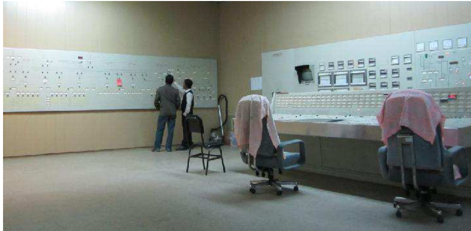
Figure 4.21: Control room at APSCL.
