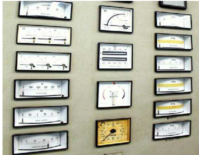
Figure 2.4: Synchroscope in the control room of 150 MW unit 3.
