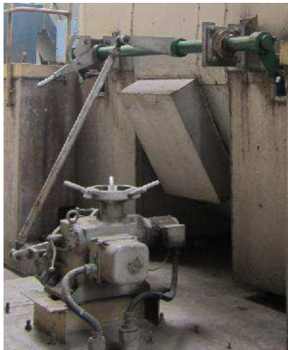
Figure 3.3: FD fan air flow control valve.
