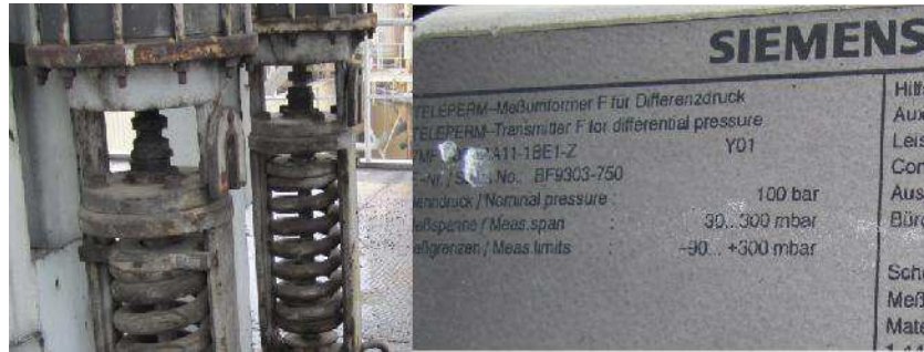
Figure 4.12: Steam pressure safety valve of boiler.
