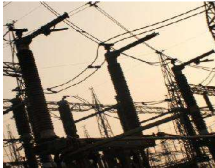
Figure 5.10: Horizontal center break isolator from APSCL.
