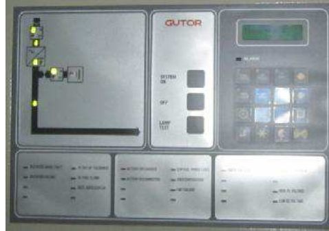
Figure 5.23: Rectifier used for battery charging purpose.
