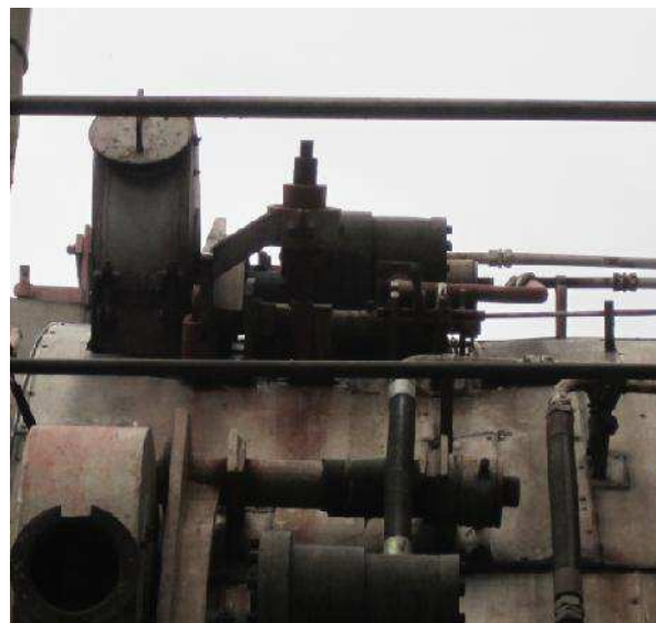
Figure 4.13: Flue gas damper of boiler.
