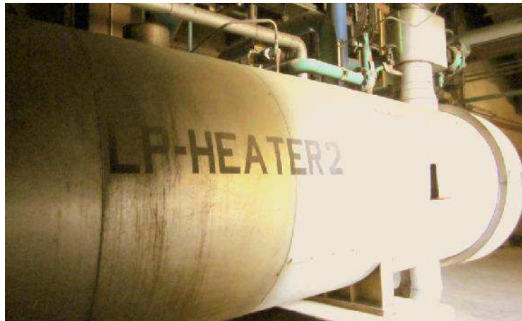
Figure 2.13: Low pressure heater in 150 MW & 15.75 KV unit 4 at APSCL.
