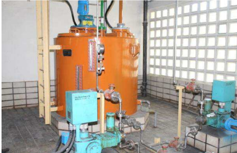
Figure 2.15: Water treatment plant in APSCL.
