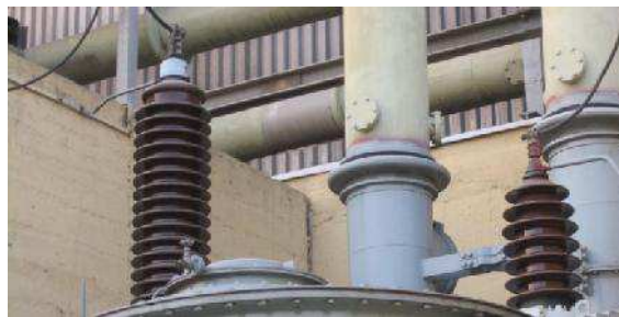
Figure 5.14: Rod gap type lightning arrester of APSCL.
