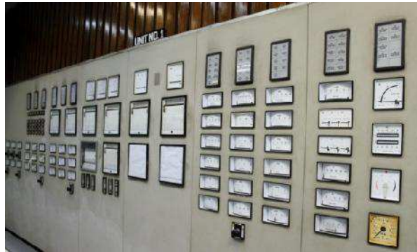
Figure 2.20: Analog monitoring parts of 64 MW & 11 KV unit 1.
