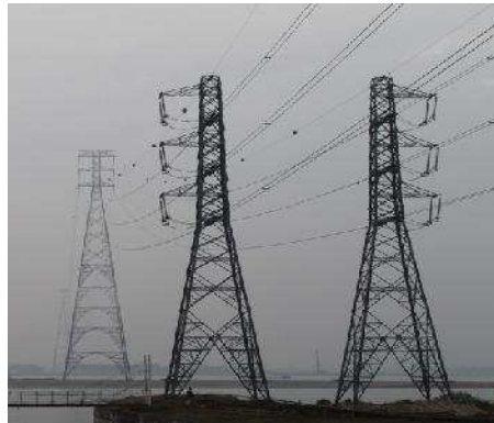
Figure 5.19: High voltage double circuit transition line.
