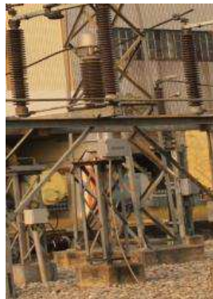
Figure 5.13: Earthing switch used in 132KV line.
