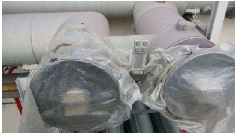
Figure 5.24: Conductors which contains 4000A current.
