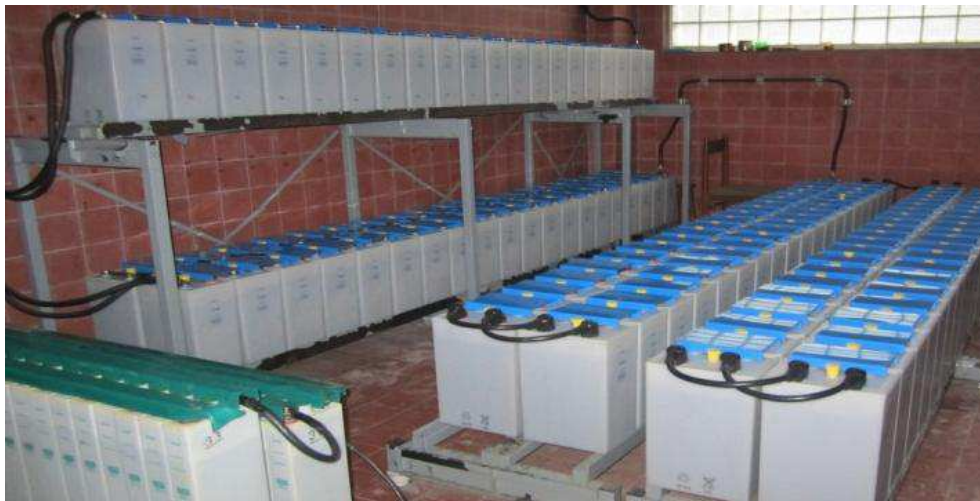
Figure 5.22: Dc battery room of APSCL substation.
