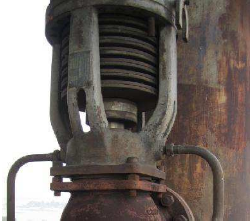
Figure 3.5: Super heater safety valve.
