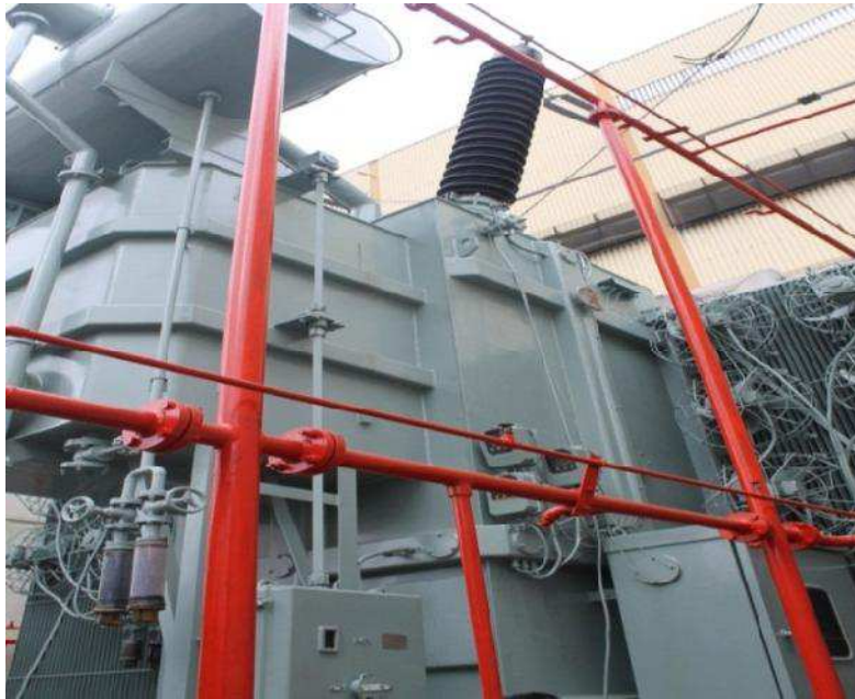
Figure 5.2: Tap changing power transformer.
