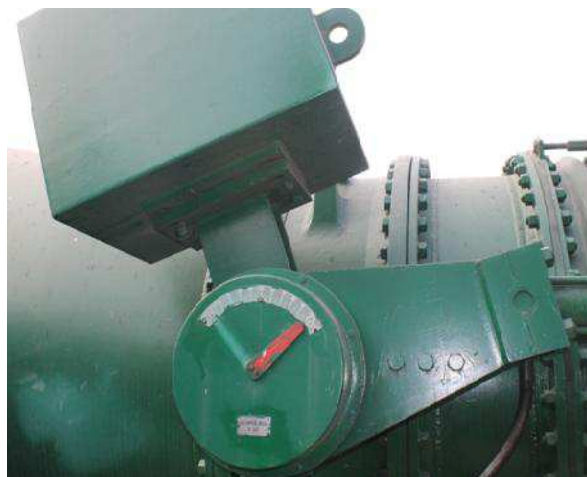
Figure 3.4: Water flow control valve.
