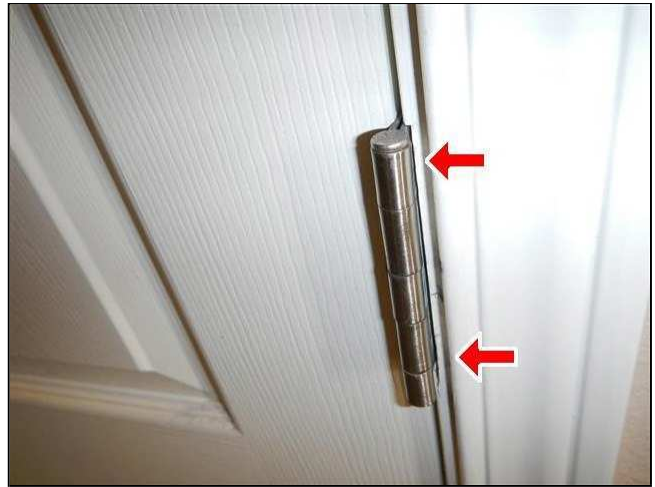
3.7 Picture 2 Bottom hinge needs repair. Screw is loose and needs a longer bigger screw in place.
