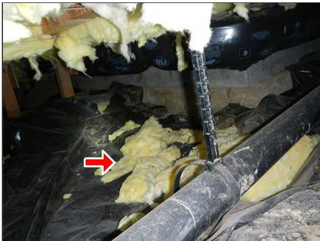
5.1 Picture 1 Some insulation has fallen, needs to be removed in order to prevent habitable locations for pests.
