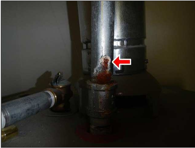
6.3 Picture 1 Small pin hole leak needs repair.
