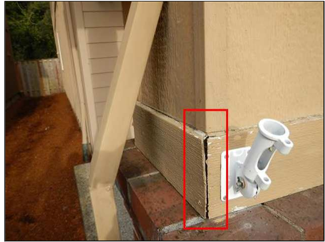
2.8 Picture 2 Cracks around trim or siding butt joints or wall penetrations should be sealed with caulking.
