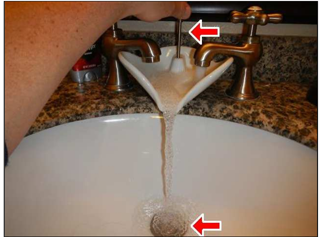
6.1 Picture 2 One pop up stopper is in need of repair. Upstairs bathroom in hallway.
