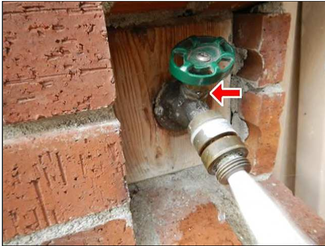
6.1 Picture 1 Both outside hose bibs leak at the stem, when turned on, and need to be repaired. This is usually an easy fix and can be repaired by replacing the internal string in the faucet.
