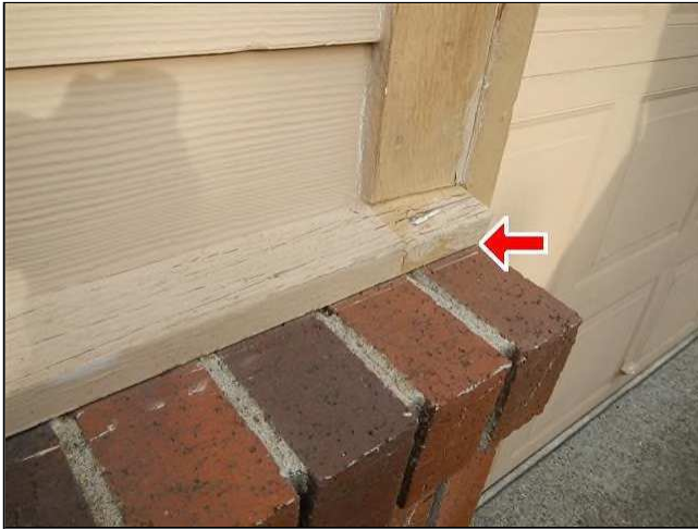
2.7 Picture 1 Paint needed on exterior of house to prevent water damage.
