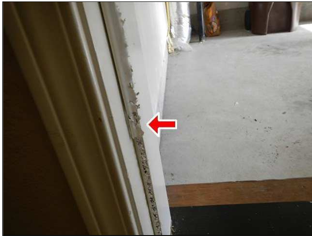
3.7 Picture 1 Weather strip, on garage door needs repair.
