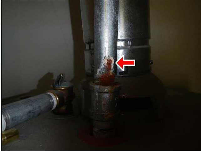
6.3 Picture 1 Small pin hole leak needs repair.
