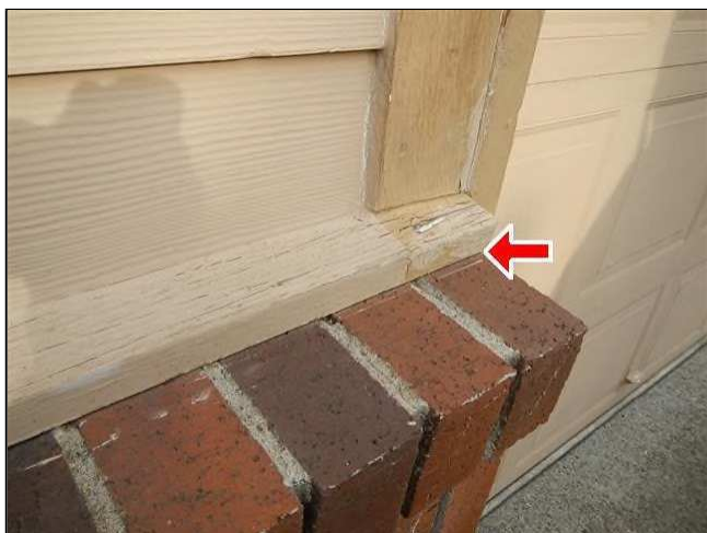
2.7 Picture 1 Paint needed on exterior of house to prevent water damage.
