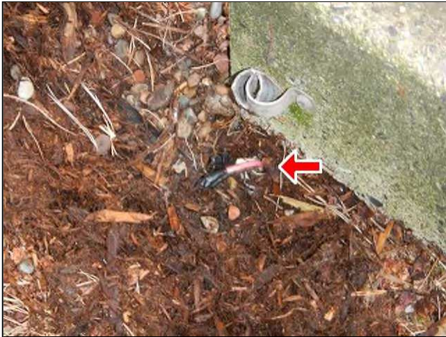
7.3 Picture 3 Dead wires coming out of ground in backyard for previous hot tub.
