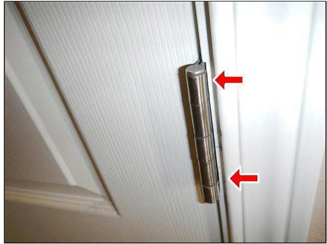
3.7 Picture 2 Bottom hinge needs repair. Screw is loose and needs a longer bigger screw in place.
