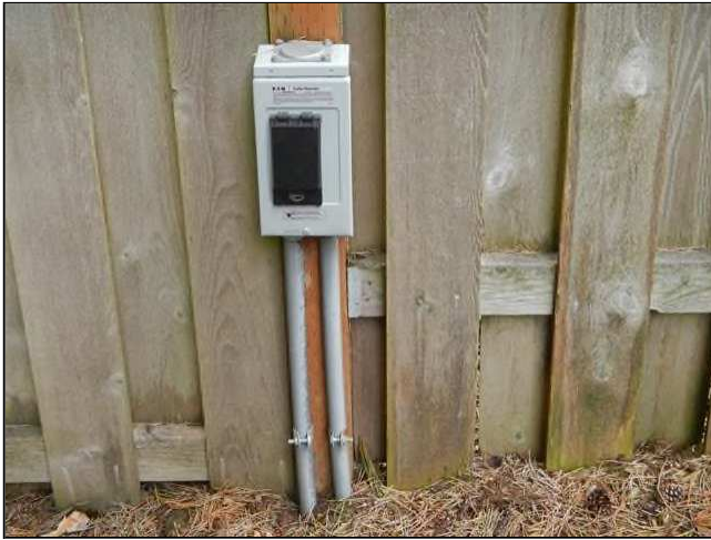
7.3 Picture 1 Outdoor 50 amp breaker for Hot tub.
