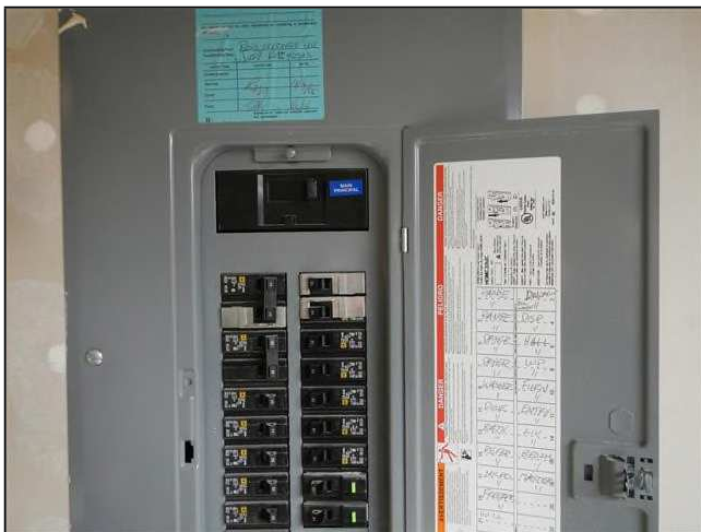
7.1 Picture 1 Properly labeled 200 amp Main Panel
