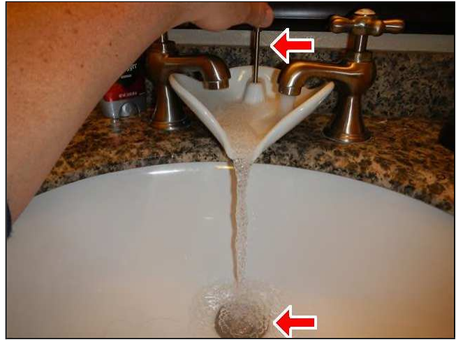
6.1 Picture 2 One pop up stopper is in need of repair. Upstair bathroom in hallway.
