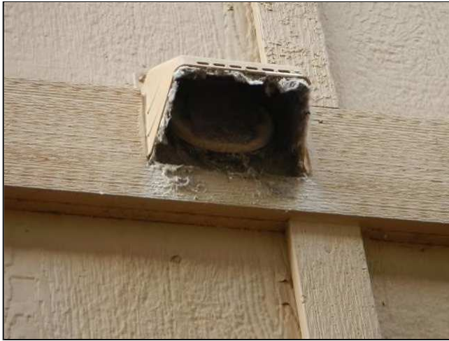
9.6 Picture 1 The dryer vent needs to be cleaned of lint. As a result, the flap is not closing properly and is a potential pest entrance to the home. Repair is recommended.
