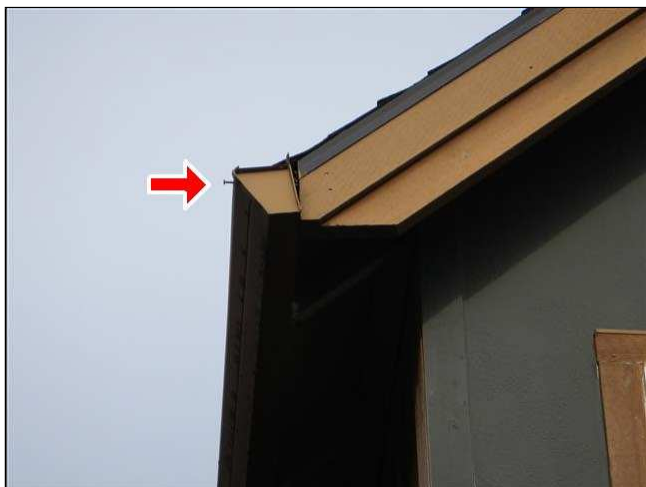
1.8 Picture 1 Spike protruding out needs to be tightened in order to keep gutter against fascia and water away from house.
