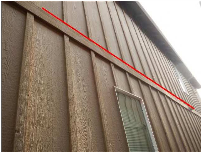
2.8 Picture 3 When repainting make sure to reapply caulking to prevent water from getting held up on top edge and getting in between board and creating water damage.
