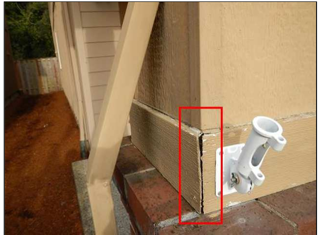
2.8 Picture 2 Cracks around trim or siding butt joints or wall penetrations should be sealed with caulking.
