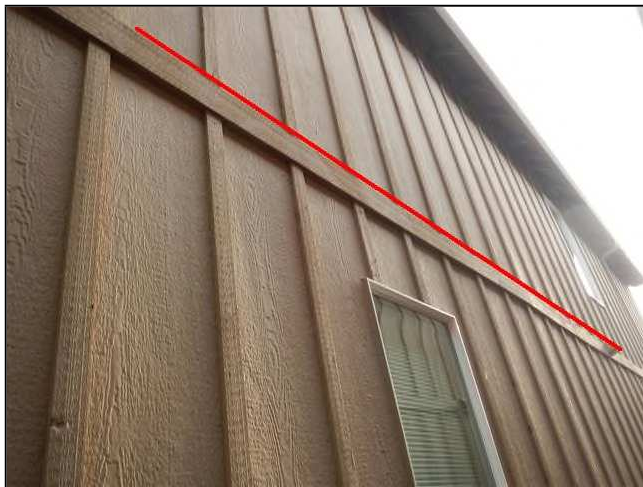
2.8 Picture 3 When repainting make sure to reapply caulking to prevent water from getting held up on top edge and getting in between board and creating water damage.
