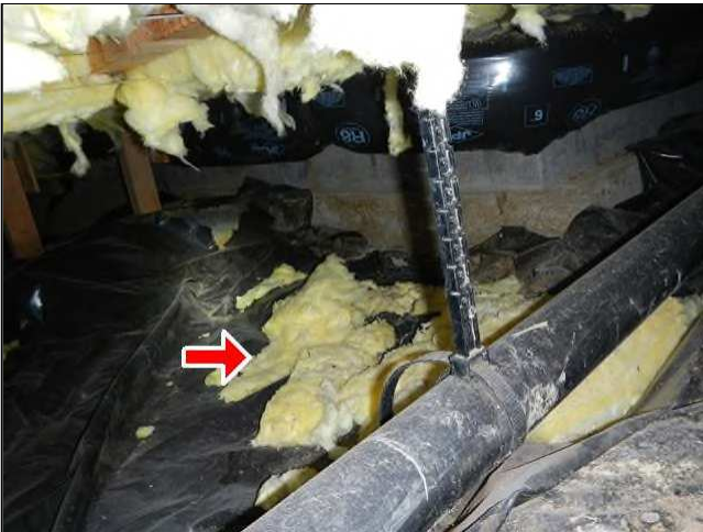
5.1 Picture 1 Some insulation has fallen, needs to be removed in order to prevent habitable locations for pests.
