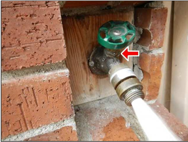
6.1 Picture 1 Both outside hose bibs leak at the stem, when turned on, and need to be repaired. This is usually an easy fix and can be repaired by replacing the internal string in the faucet.
