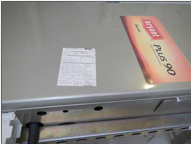
8.0 Picture 1 There are no maintenance documents on the furnace. If it has not been serviced within the last two years, servicing by a n HVAC company is recommended. In particular, the heat exchanger should be checked for possible cracks.
