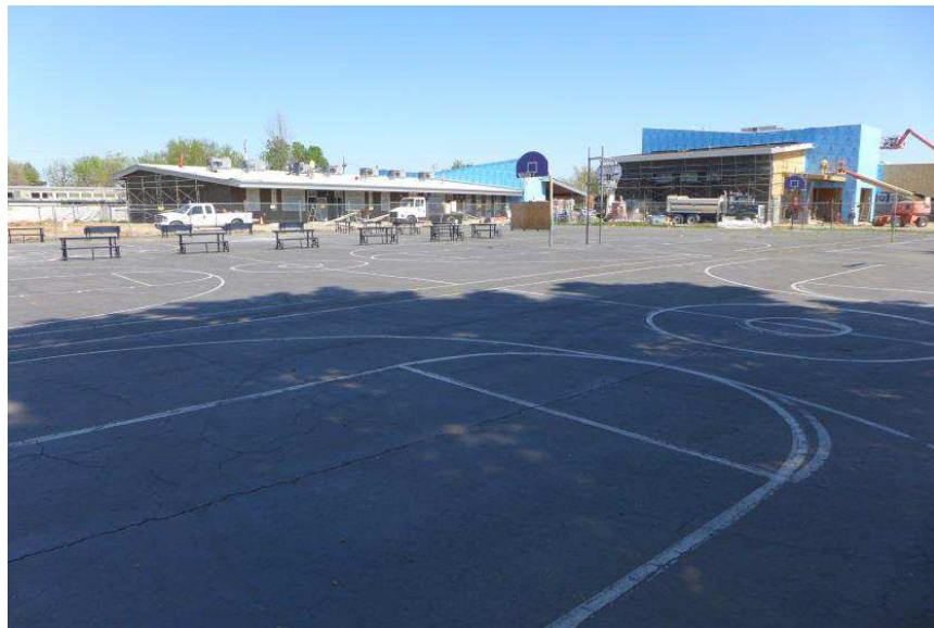
Construction on Main Avenue's new classroom facility (left) and cafeteria (right). (Credit: CFW, Inc.)
