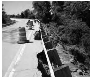
Drums warn motorists of a washed-out road.
