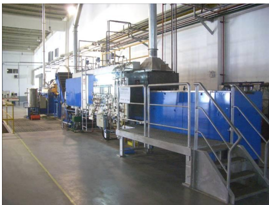
Figure 4 Mesh Belt Furnace
