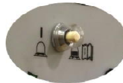
Disconnected circuit breaker
