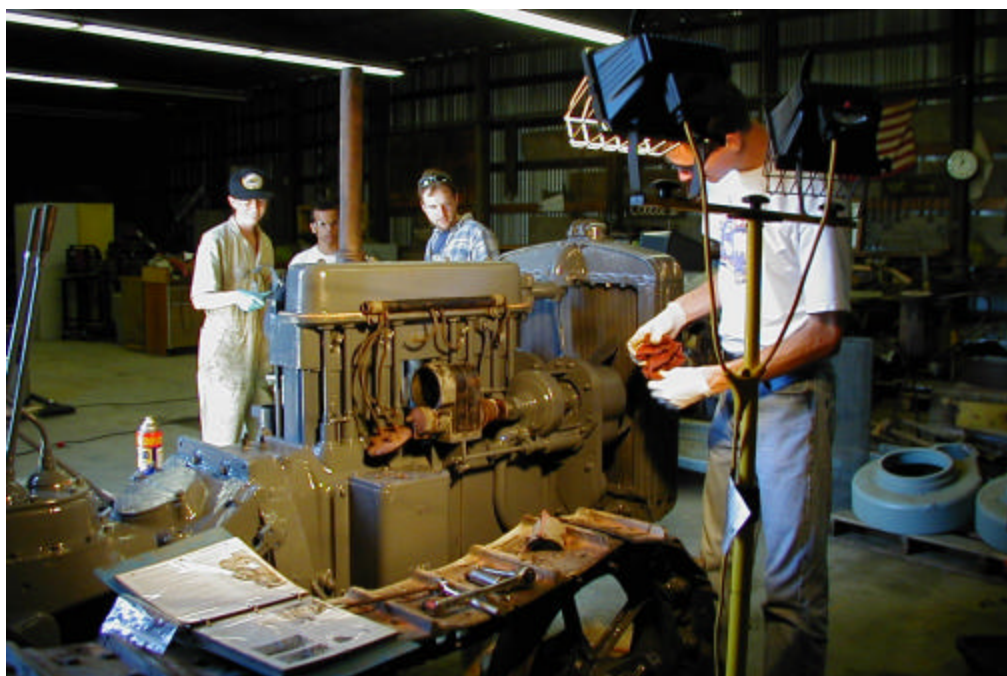
Shedding some light on the situation: Jim Keller installs and times the magneto on the Caterpillar Twenty, while Sue Esdaile, Mikko Solomon and Jacob Chapin look on.
