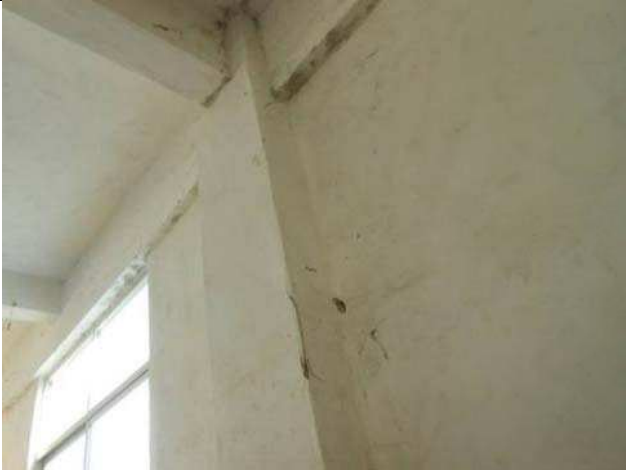
NC:1.2/7.5 The dirty cobwebs were found in packing area and finished product warehouses.
