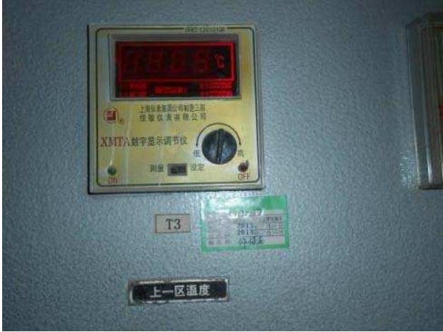
Temperature monitor device with calibration label
