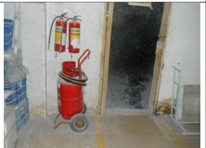
Extinguisher in workshop
