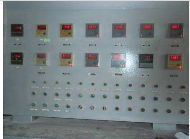
Kiln control panel
